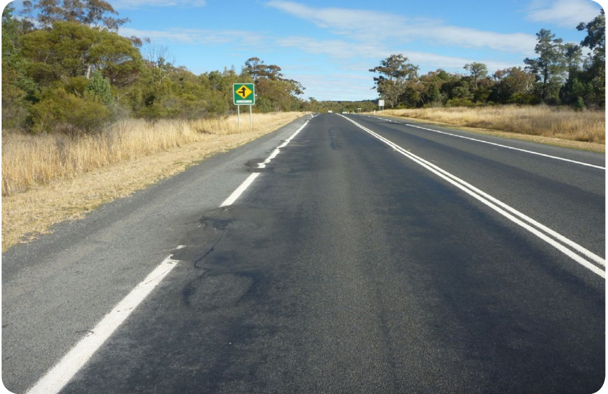
Pavement deterioration south of Dubbo
