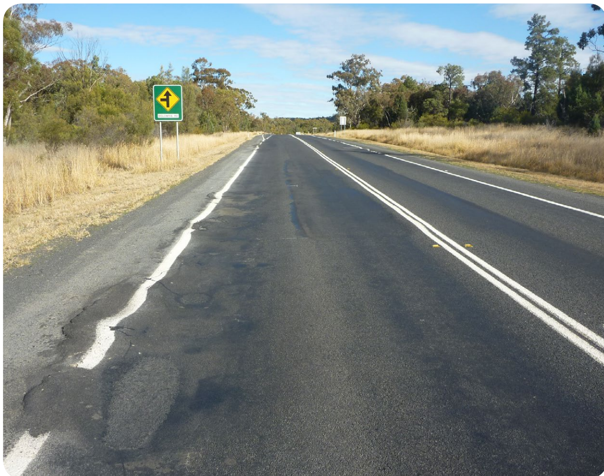
Typical pavement deformation on the Newell Highway
