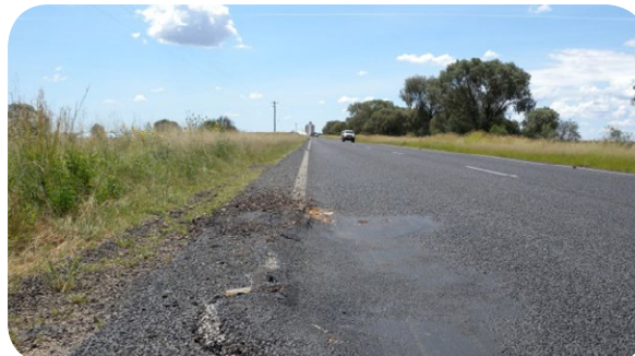
Typical edge pavement failure
