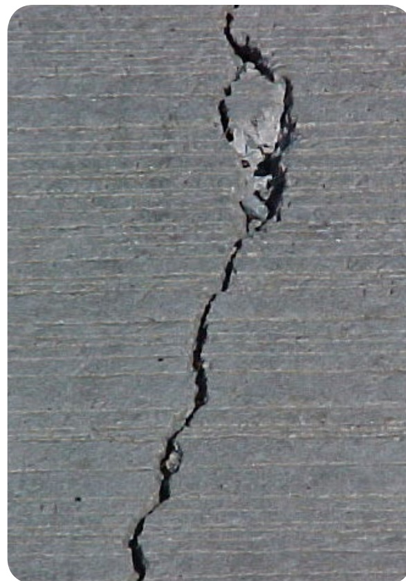
Large pavement cracking
