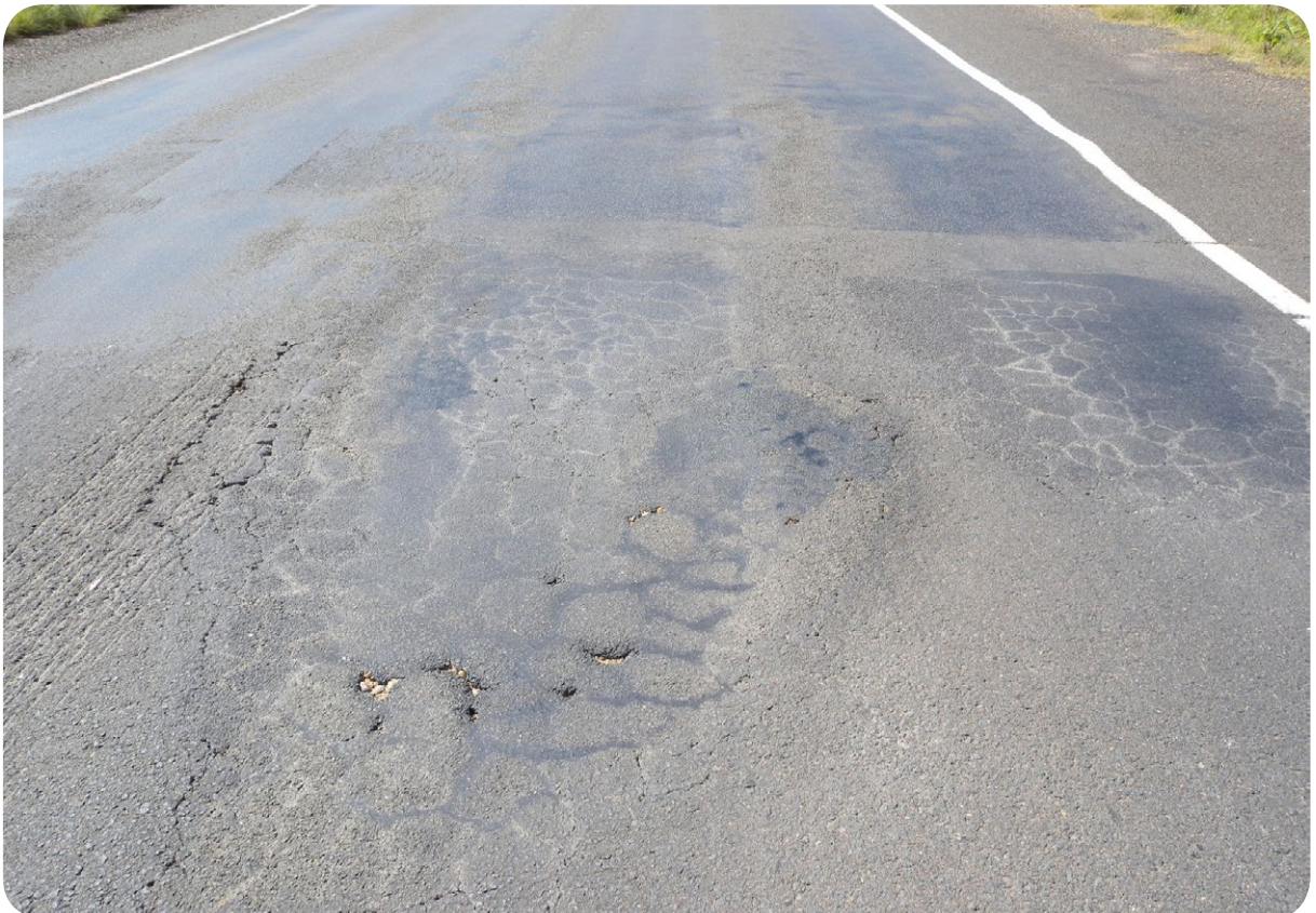
Typical pavement cracking
