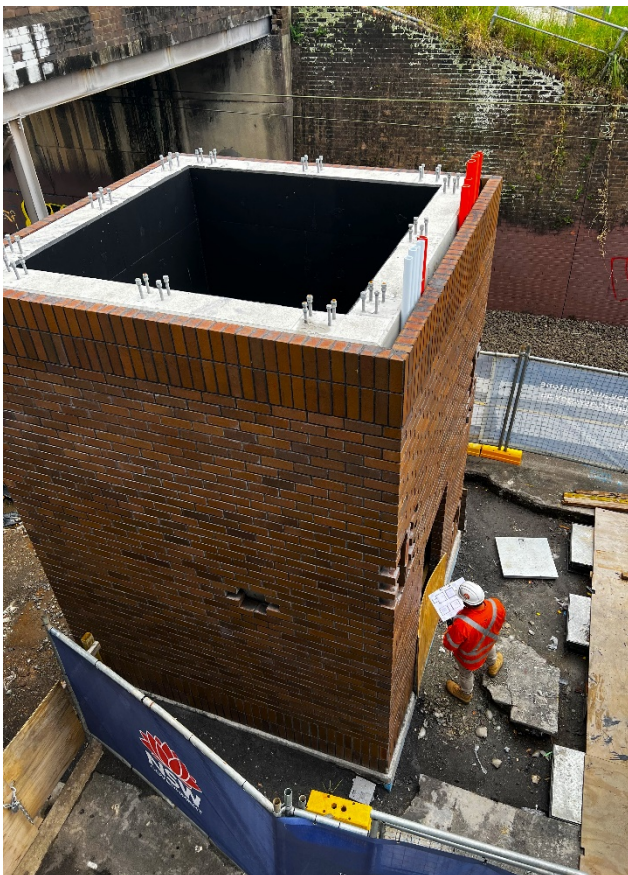
Behind the scenes: works are progressing on upgrading the station facilities, which includes installing lifts to improve station access
