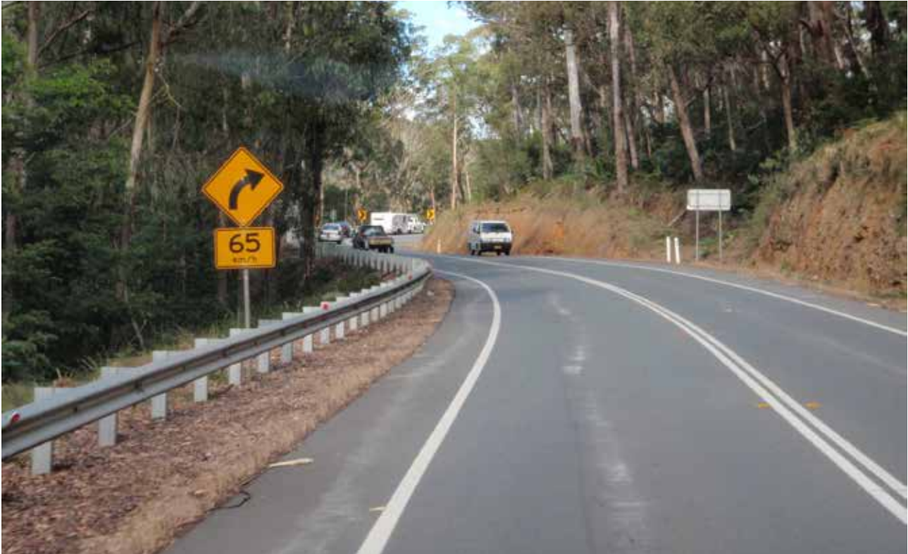
Photograph 2.10: Misleading curve warning sign
