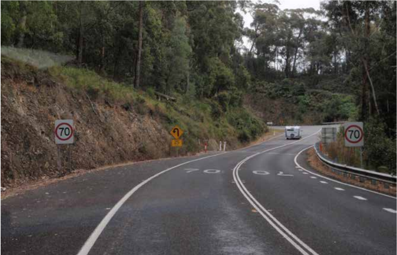
Photograph 2.12: Poorly placed speed zone signs
