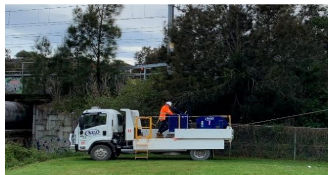
Cable installation truck used during work on Saturday 16 July and Sunday 17 July
