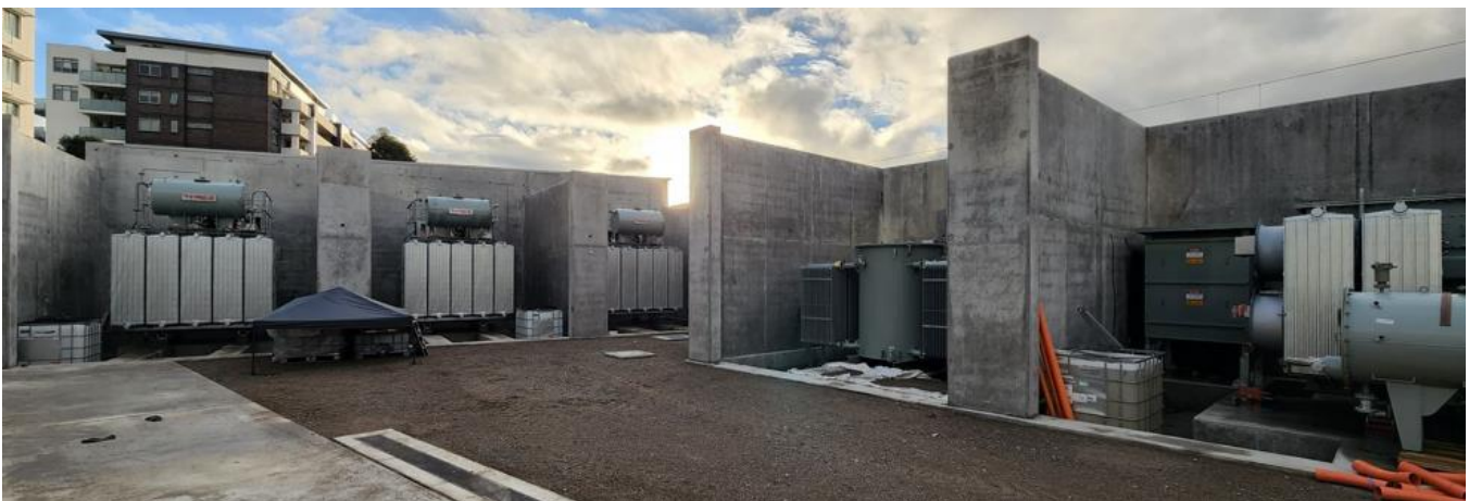
Newly installed substation power transformers at the substation site
