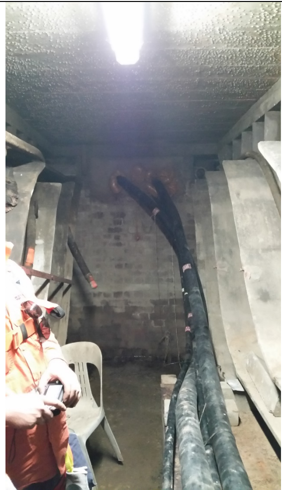
Plate 4 Service pit and tunnel showing past cable egress impacts to the brick wall
