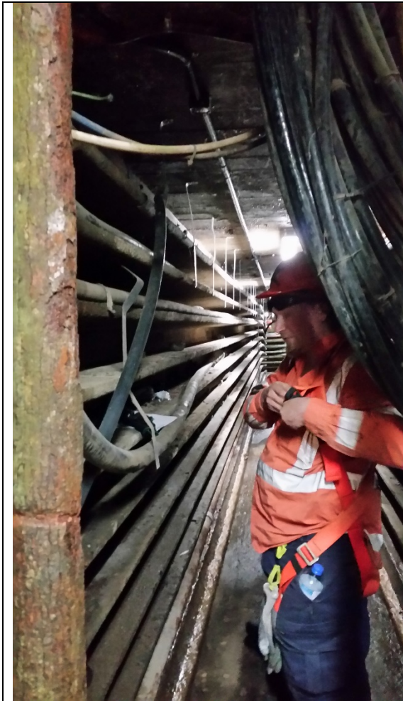
Plate 3 Service pit and tunnel with existing cables
