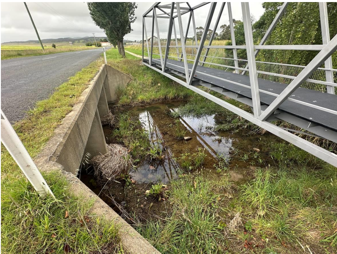
Photo 4: Southern culvert downgradient of site fence line with surface water flowing offsite. Surface water is clear with a slight brown tint and low to no turbidity.
