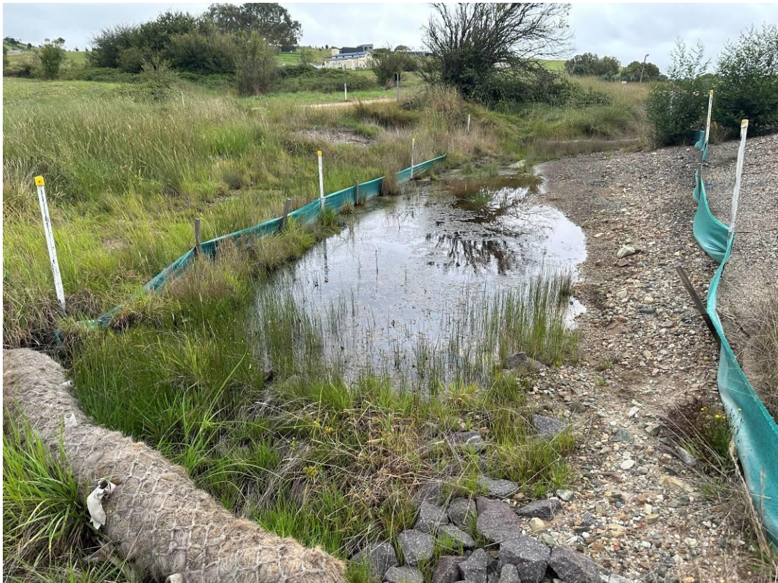
Photo 14: Surface water pooled upgradient of railway line. Sediment controls (coir logs, silt fencing and rock armoury) in place and adequate. Surface water was clear with low to no suspended solids.
