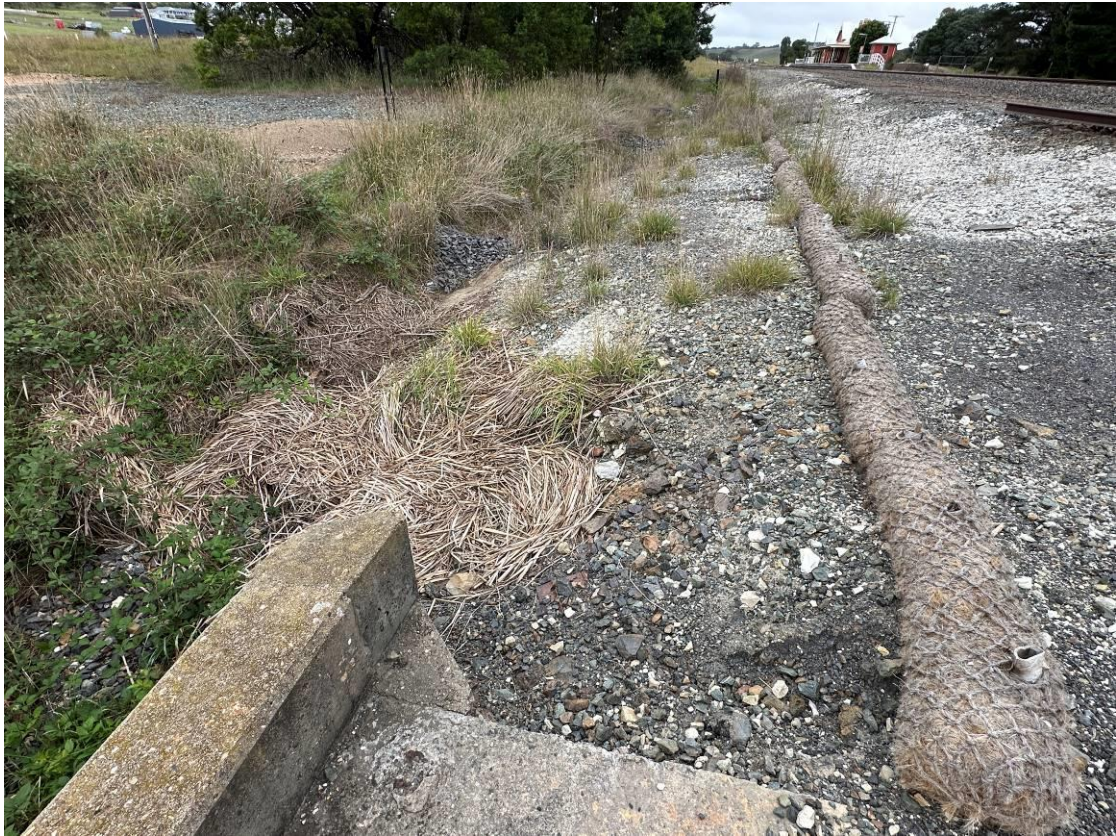
Photo 9: Southernmost culvert upgradient of the railway line. Evidence of previous high surface water flow (build-up of vegetation debris). Sediment control coir logs in place and in good condition.
