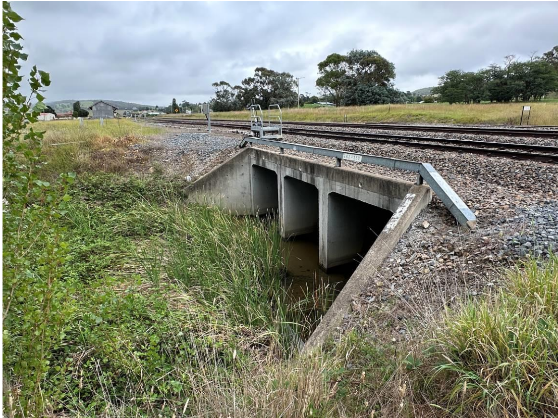
Photo 3: Southern culvert downgradient of railway line with surface water flowing offsite. Surface water is clear with slight brown tint and low to no turbidity.
