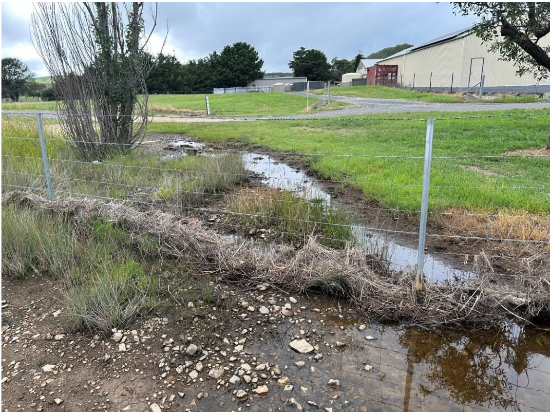
Photo 6: Downgradient of middle culvert facing east with flowing surface water. Surface water across road causeway appeared clear with low turbidity and suspended solids.
