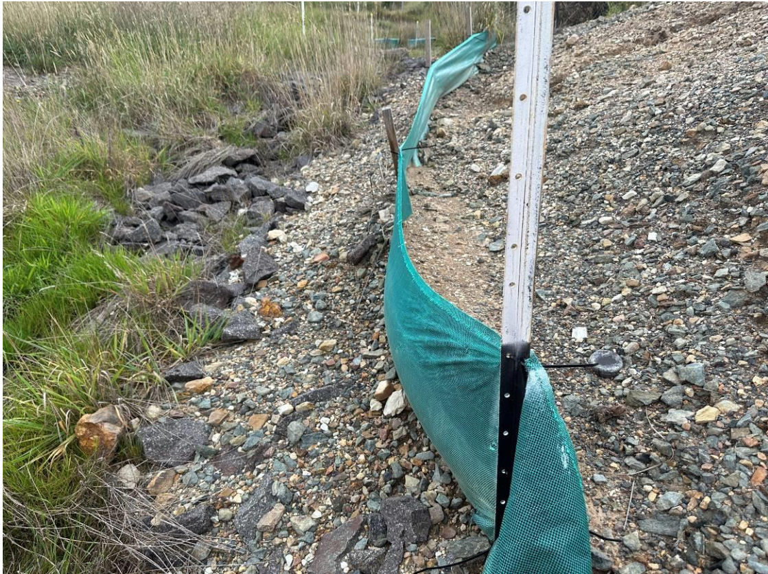
Photo 15: Upgradient of railway line to the north of the middle culvert. Sediment fencing in place with large build-up of sediment.
