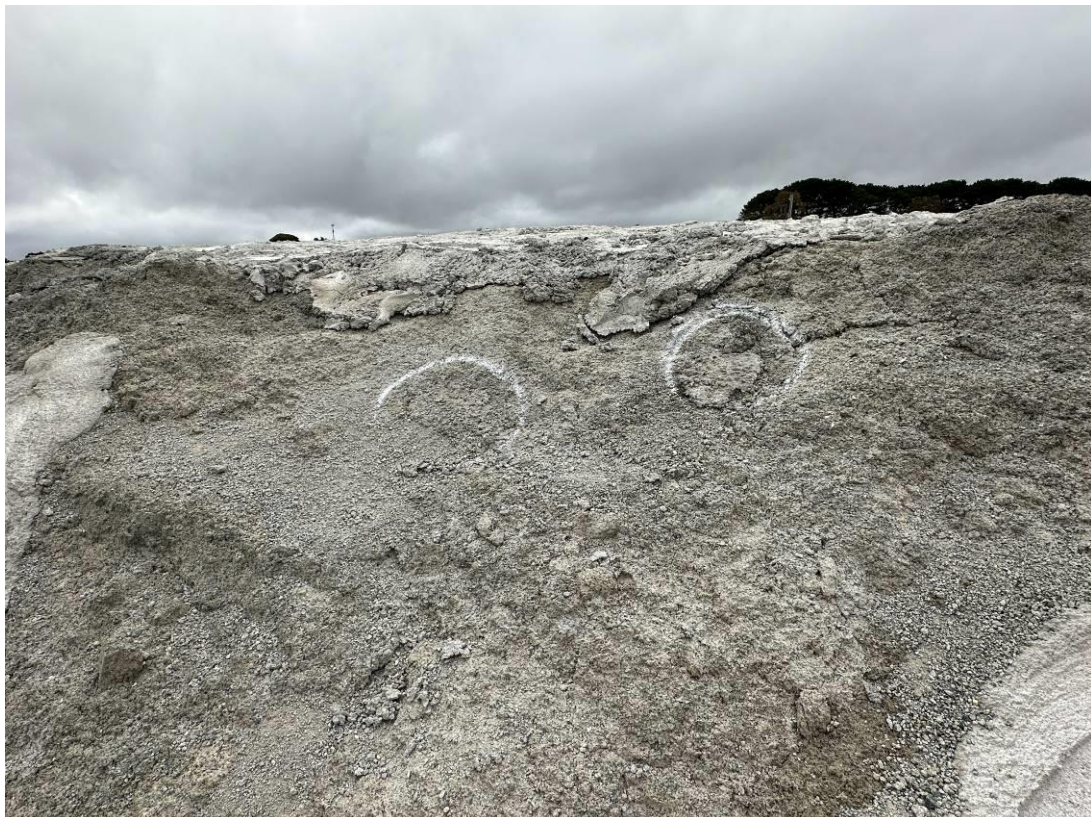
Photo 16: Exposed geofabric layer marker on stockpile (identified during the January inspection) has since been filled in with concrete.
