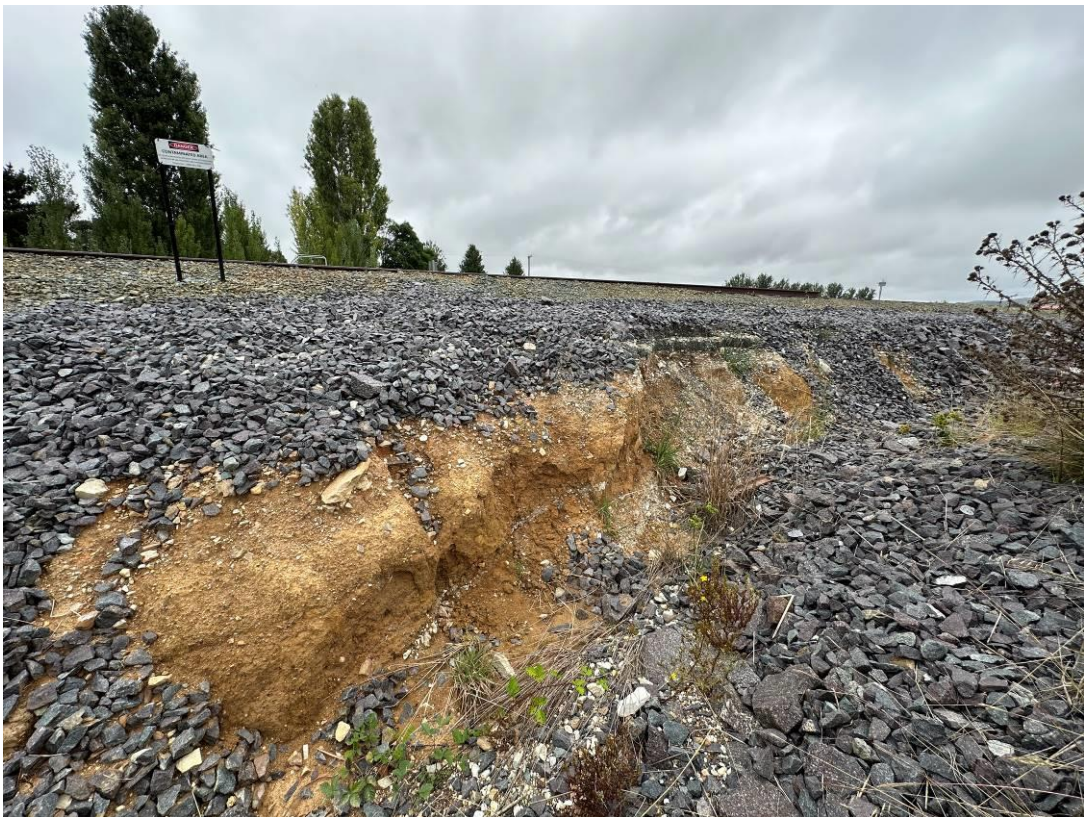
Photo 10: Southernmost culvert upgradient of the railway line. Evidence of erosion due to lack of ground cover. Only minor changes since previous inspection.
