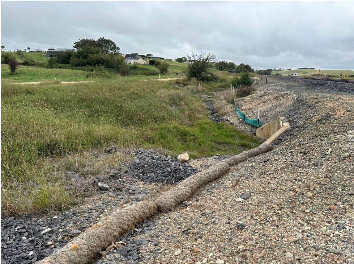
Photo 11: Upgradient of middle culvert. Sediment controls in place (coir logs and rock armoury in good condition).
