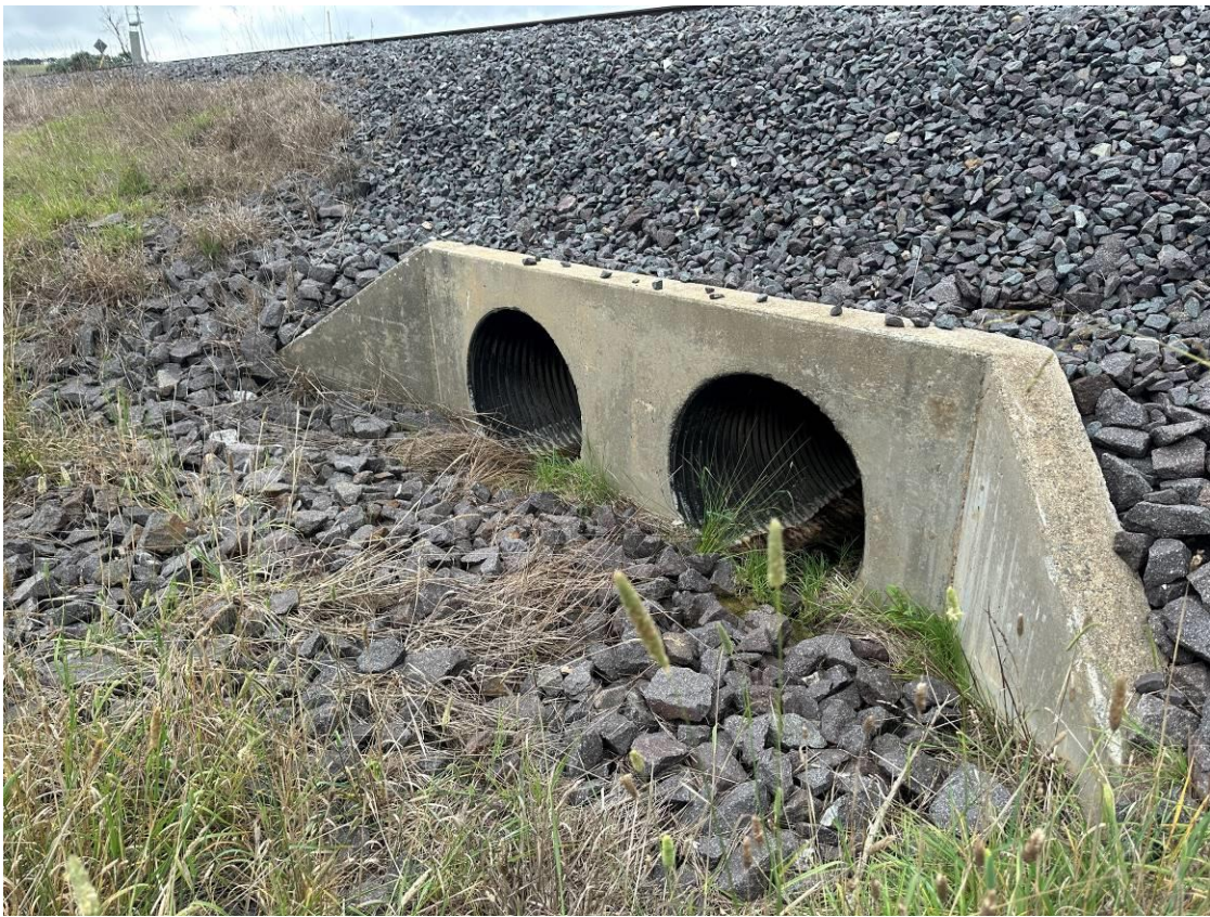
Photo 13: Upgradient of northernmost culvert with no surface water. No sediment build up was noted on rock armoury.
