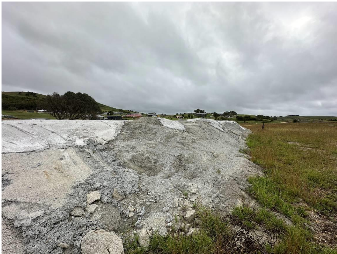
Photo 17: Concrete capped stockpile. No new signs of exposure marker layer and erosion damage.
