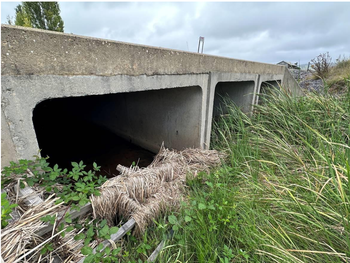
Photo 8: Southernmost culvert upgradient of the railway line with flowing surface water. Evidence of previous high surface water flow (build-up of vegetation debris).
