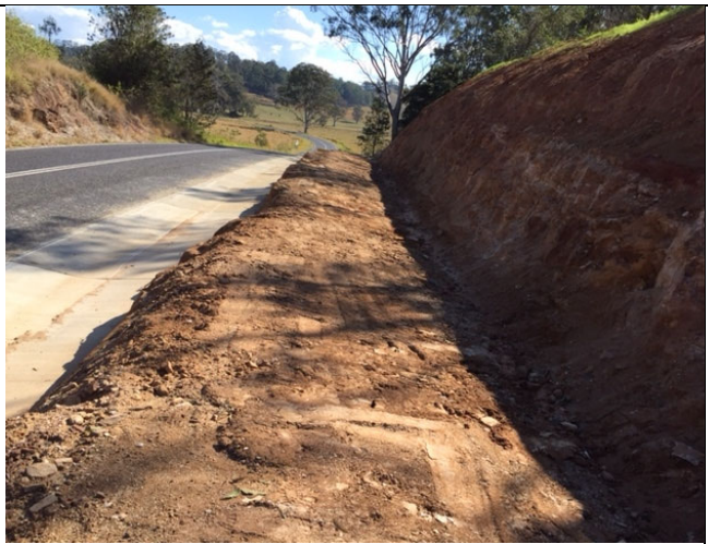
Pic 4 – Typical shoulder widening of cut batter and berm and replacement of SO gutter
