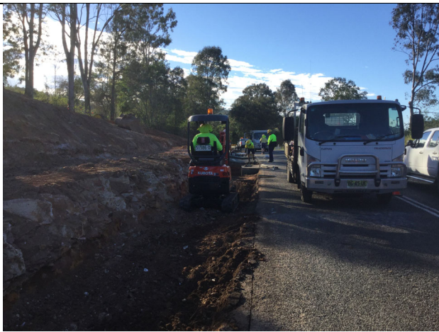
Pic 3- Typical excavation of existing table drain subgrade and replacement with select material
