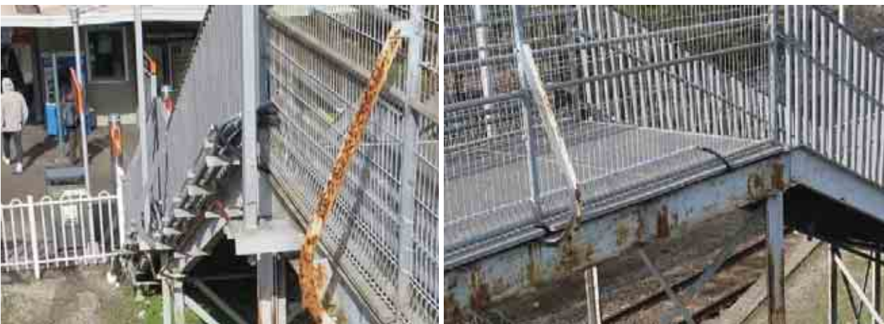
Figure 2-9: a) LEFT: View of services on eastern side of central stairs (lighting, signalling and communications), b) RIGHT: View of service from Pacific Highway crossing from western to eastern side of central stairs (Telstra)
