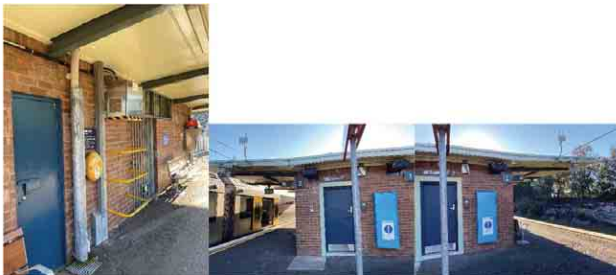
Figure 4-52: Telstra Wi-Fi System
