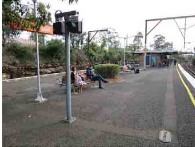
Figure 2-15: Existing back-to-back Guard Indicator on Up Platform (Platform 1)
