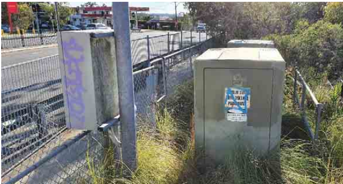
Figure 4-20: Existing 30kVA padmount 415/415V isolation transformer supplying station DB
