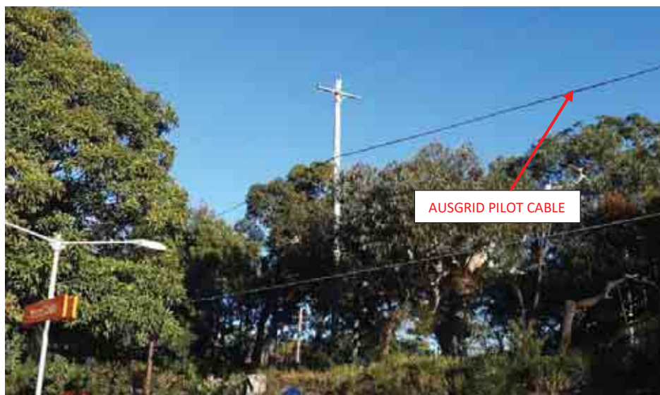
Figure 2-6: Photo of Ausgrid Pilot Cable Attached to Pole No.25
