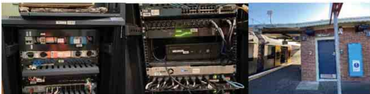
Figure 4-48: View of PA rack and platform speakers City end of existing station building
