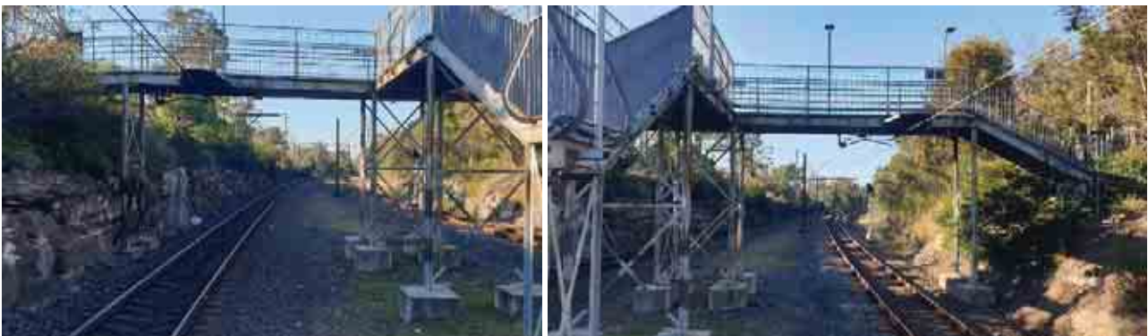
Figure 2-2: View of existing footbridge from Platform a) LEFT: Span over Down Main, b) RIGHT: Span over Up Main
