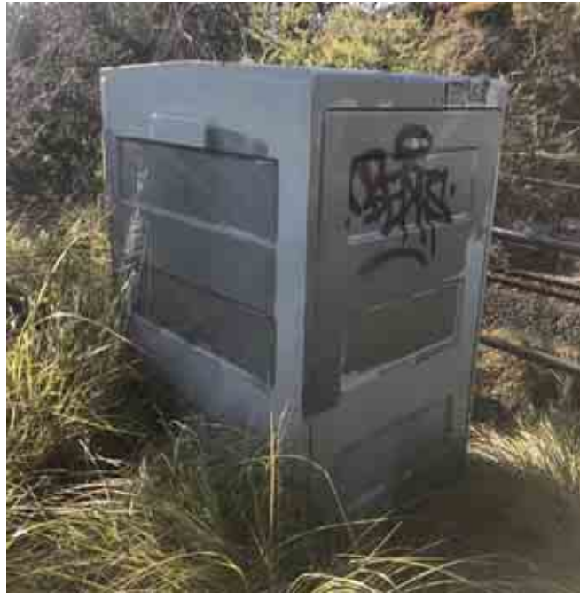
Figure 4-26: Existing backup signaling padmount substation 5kVA 240/120V
