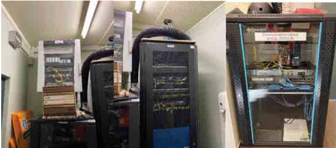
Figure 2-11: Existing services rack in station building
