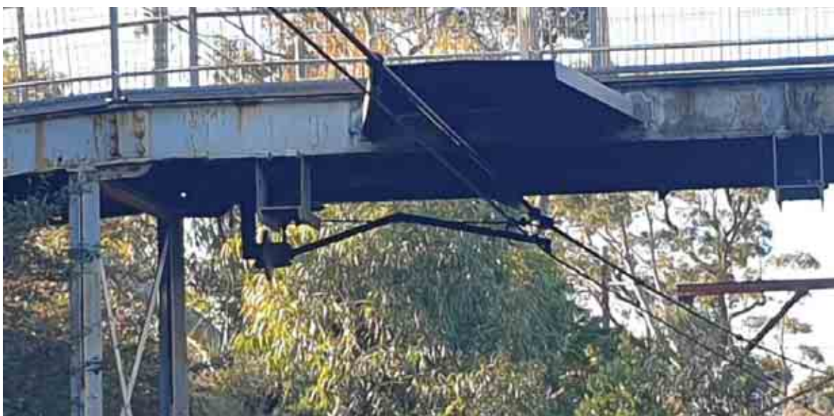
Figure 5-12 View of existing metal structures - OHW (from Down Side platform, facing north)
