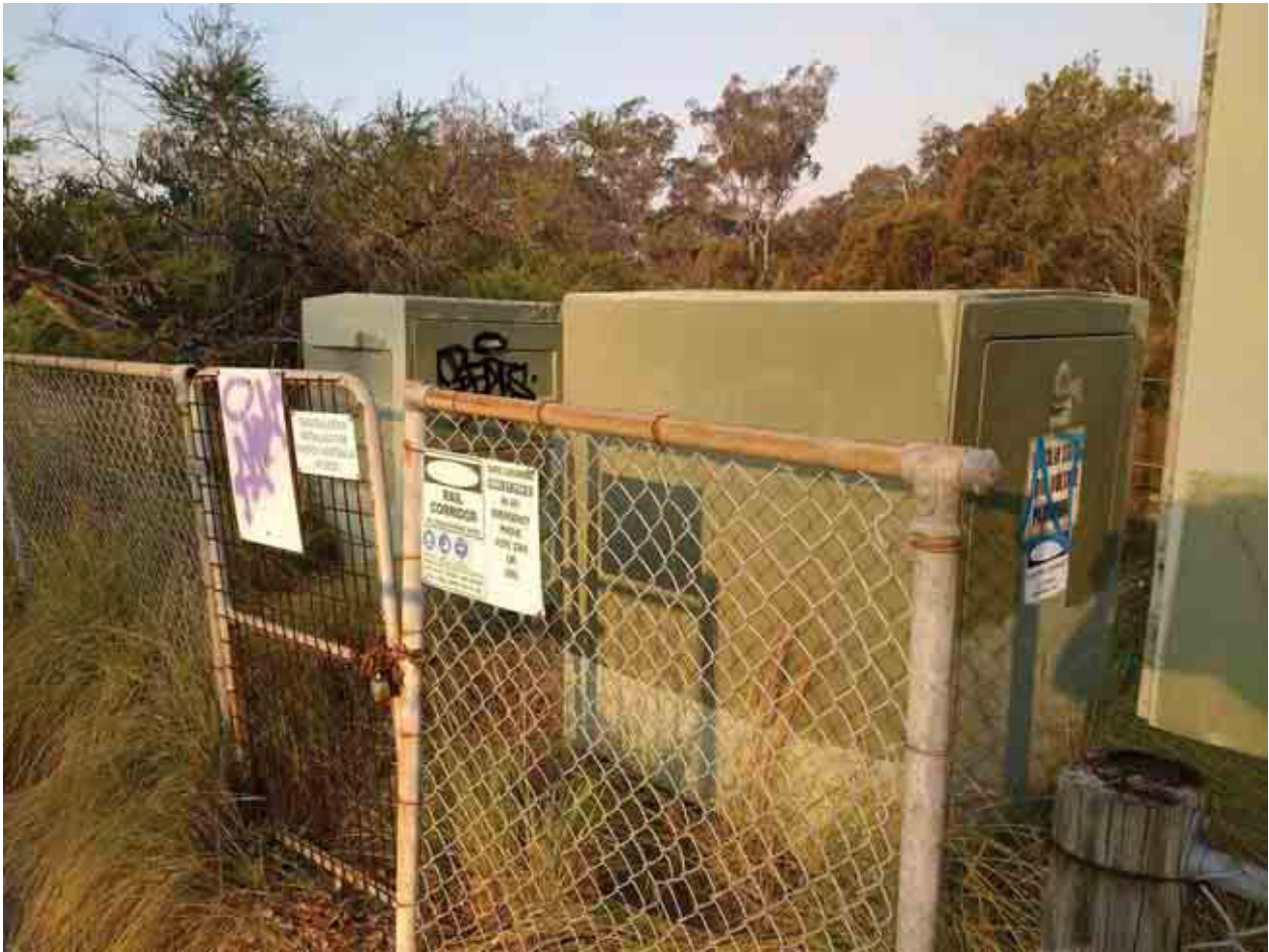
Figure 5 Private Padmount Isolation Transformers for Main Station and Backup Signalling Loads
