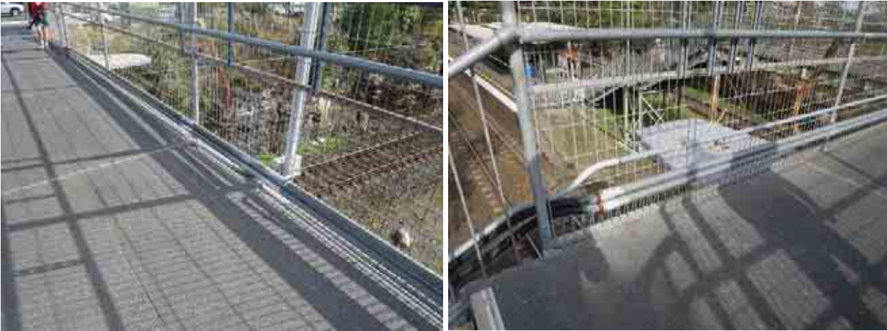
Figure 2-8: a) LEFT: View of existing services on Country side of existing footbridge (power supply); b) RIGHT: View of services from Signal Loc N23.48R on City side of existing footbridge (signalling and communications)
