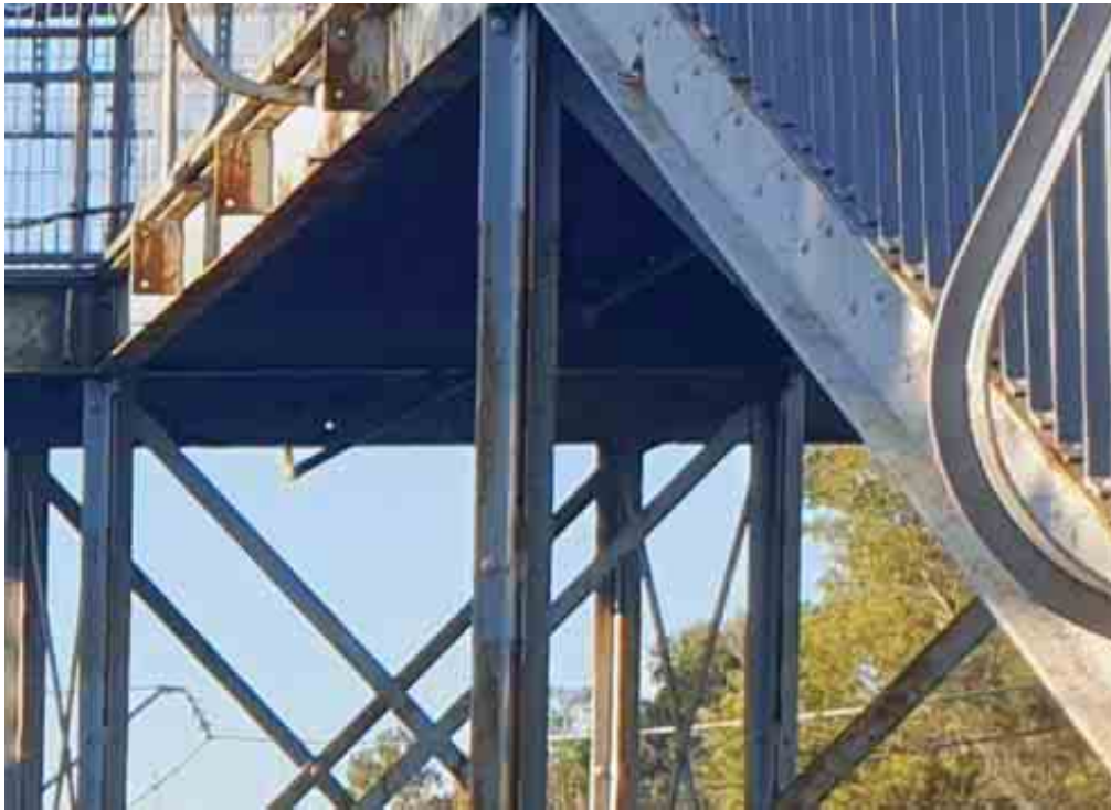
Figure 5-11 View of existing metal structures under the stair case - unsuitable microbat habitat (from Down Side platform, facing north)
