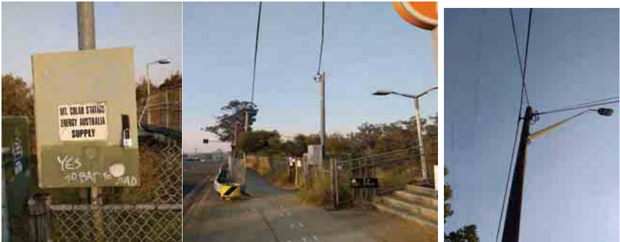
Figure 2 Existing Ausgrid Supply via a private pole fed from Ausgrid Pole MC-2343 on Pacific Highway
