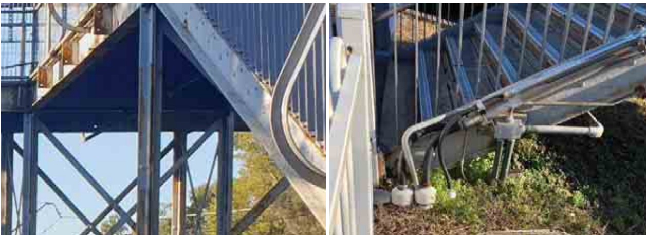
Figure 2-10: a) View of services running below existing footbridge (station power supply), b) View of services at bottom of central staircase (signalling and communications, LV)
