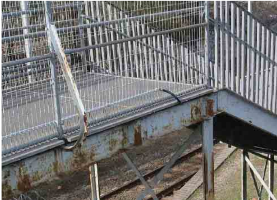
Figure 5-13 View of existing metal structures from Pacific Highway side of footbridge - unsuitable microbat habitat
