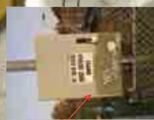
Mt Colah Station Ausgrid Supply
