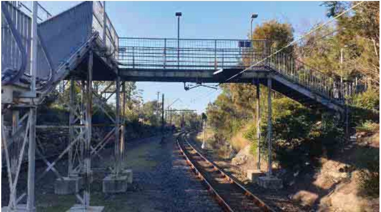
Figure 2-5 View of existing footbridge from platform (Up Main, facing north towards Country)
