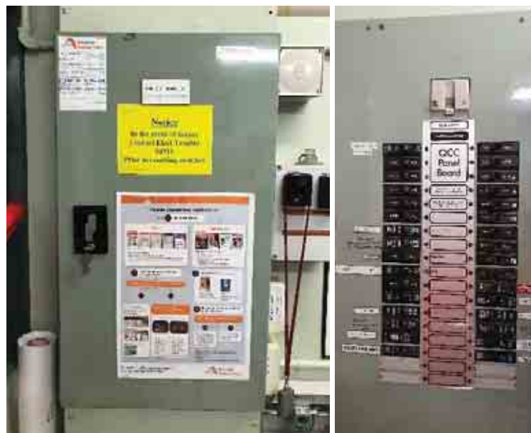
Figure 4-21: Existing Station DB
