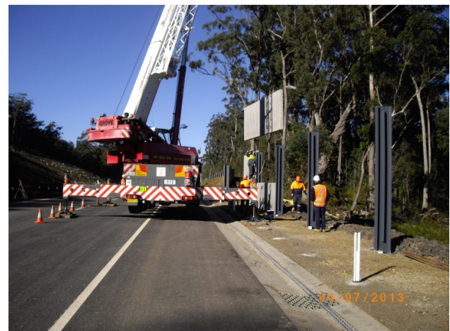
Pacific Highway Upgrade – Bulahdelah Bypass: Noise wall panels being lifted in using a mobile crane.
