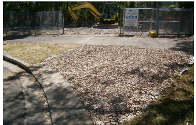
Figure 8: Stabilised access point constructed from geo-fabric and recycled concrete to facilitate access to site along nominated local roads. Stabilised access points are maintained during construction and removed when no longer required. Source: M5WW Project.
