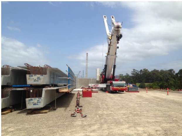
Pacific Hwy Upgrade – Oxley Hwy to Kundabung: installing bridge girders from reinforced earth walls (soil walls)
