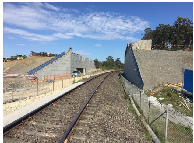
Pacific Hwy Upgrade – Oxley Hwy to Kundabung: reinforced earth walls (soil walls) nearing completion.
