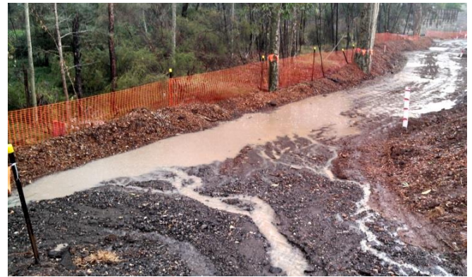
Figure 1: Mulch bund utilised on the M5WW project to manage construction runoff. Source: M5WW Project.
