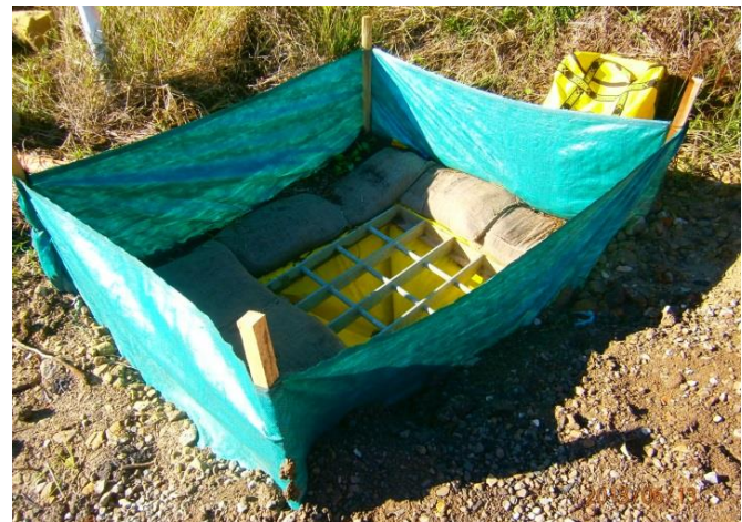
Figure 3: Triple controls installed to protect inlet pits along the M5WW project comprising of sediment fence, sandbags and a pit bag. Source: M5WW Project.
