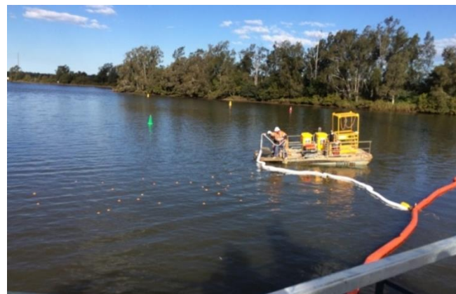
Figure 19: Emergency spill response procedures being tested at the Oxley Highway to Kundabung Project over a waterway. Source: Oxley Highway to Kundabung Project.
