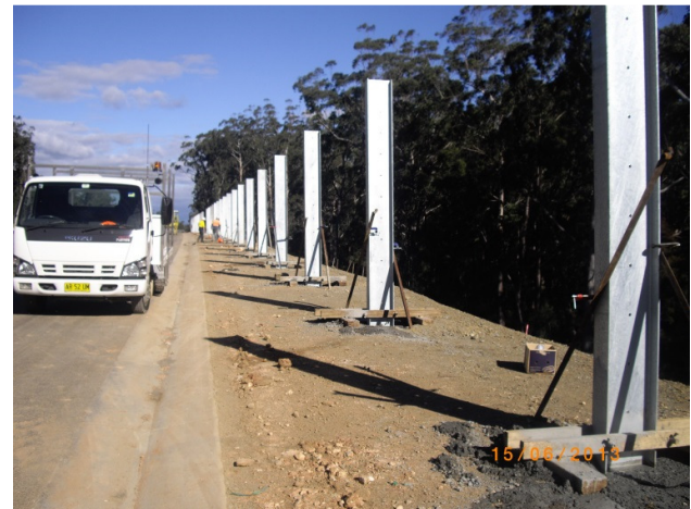
Pacific Highway Upgrade – Bulahdelah Bypass: Noise wall post installation after embankment construction.
