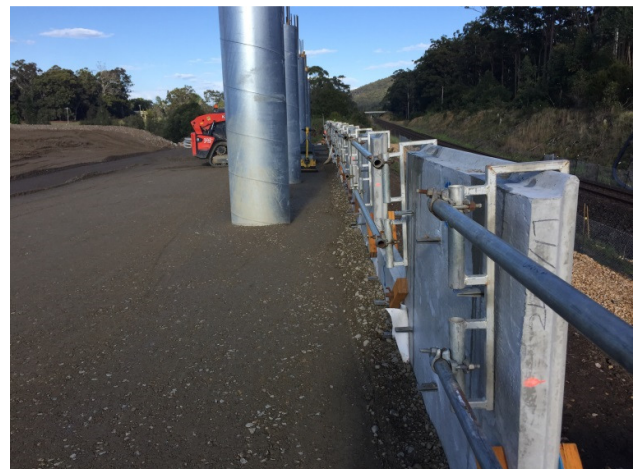
Pacific Highway Upgrade – Oxley Hwy to Kundabung: construction of reinforced earth walls (soil walls) around sleeved column extensions.
