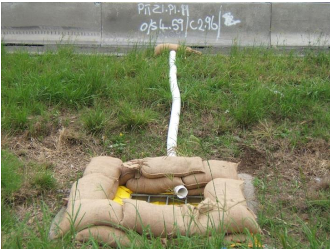
Figure 6: Temporary diversion pipe to divert clean water from the carriage directly into the stormwater network while working in the median. This reduced the amount of construction runoff within the median that required treatment. Source: M5WW Project.
