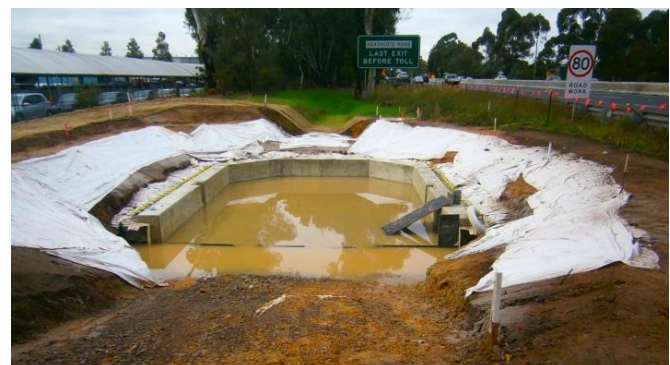
Figure 4: Operational basin utilised to collect construction runoff during construction following consultation and approval from the EPA. Source: M5WW Project.
