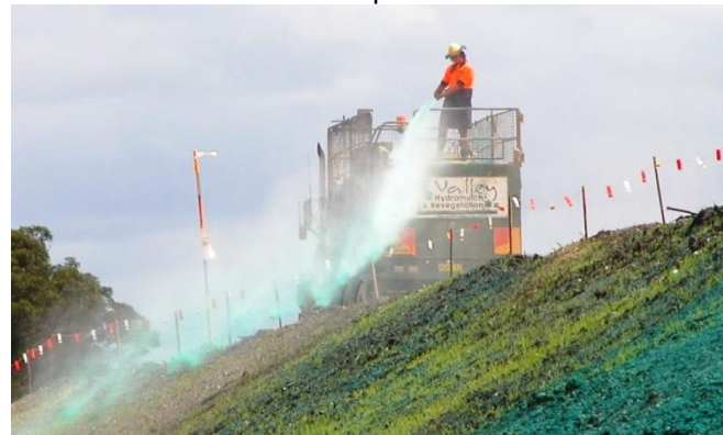
Figure 7: Stabilisation of exposed batters to prevent erosion and dust impacts. Source: NH2U.
