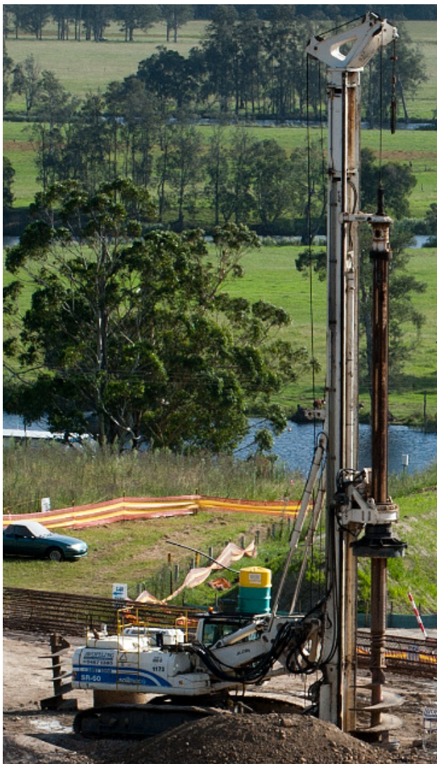
Pacific Hwy Upgrade – Bulahdelah Bypass: Construction of 1200mm bored piles for Myall River Bridge Abutment
