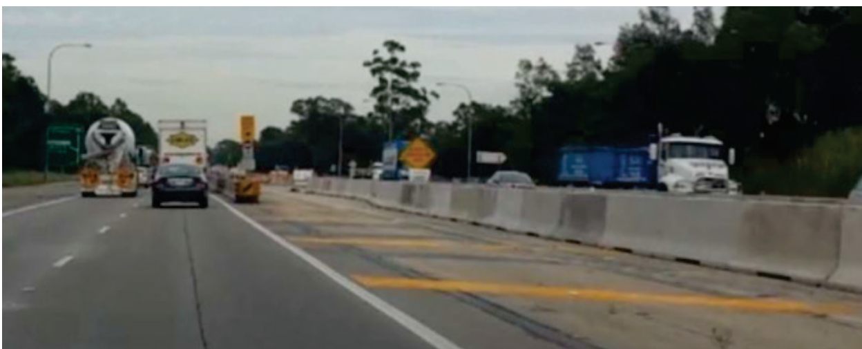
Example of a typical gate arrangement, for carrying out pavement construction works, between live traffic. Source: M5WW.
