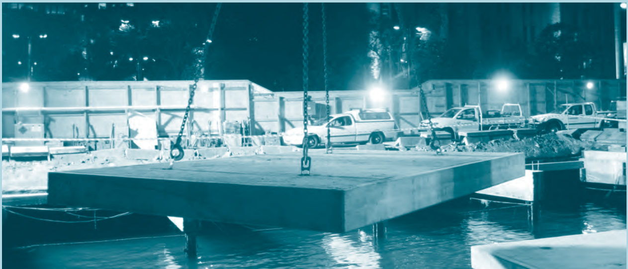
Replacement of skirting and deck panels on the western promenade of Circular Quay were completed during the year.
