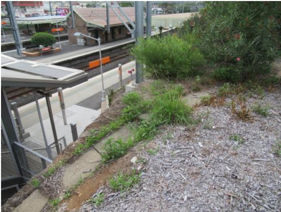
Photo 4: GLT at top of failed section
