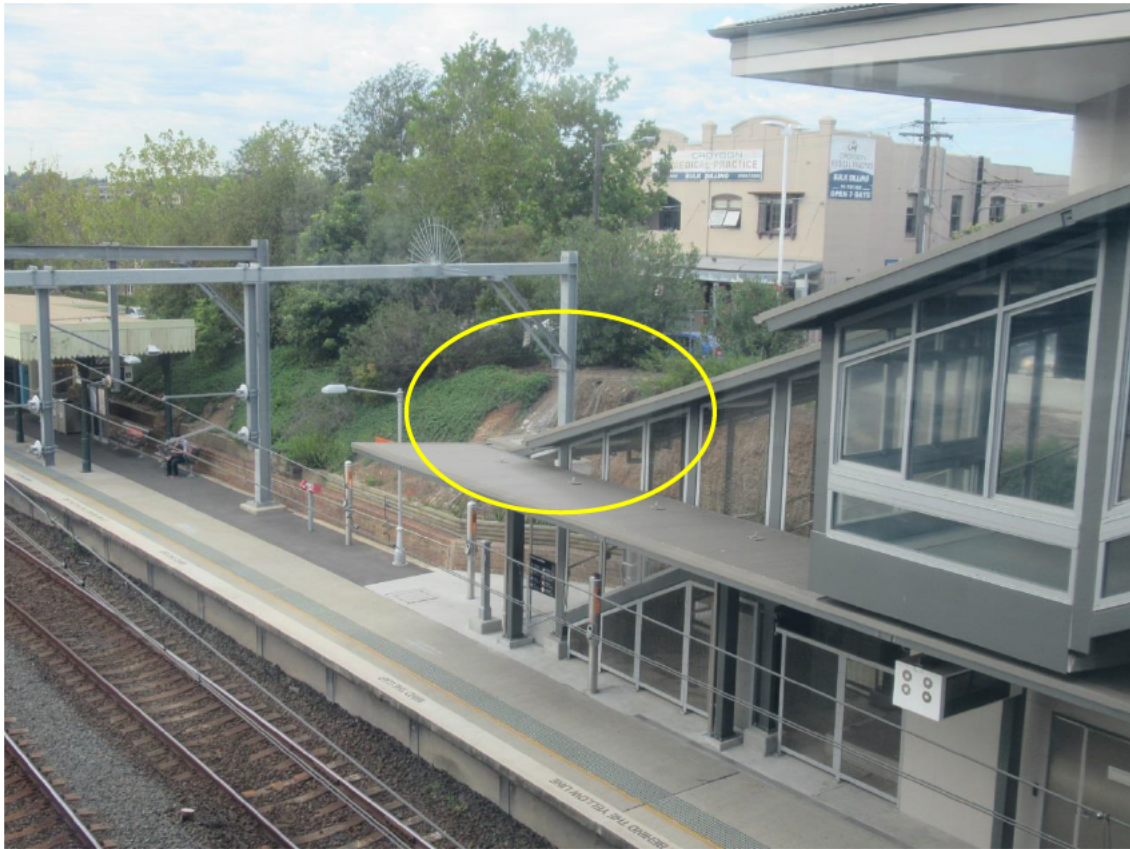
Photo 1: Location of the failed section adjacent to Platform 5
