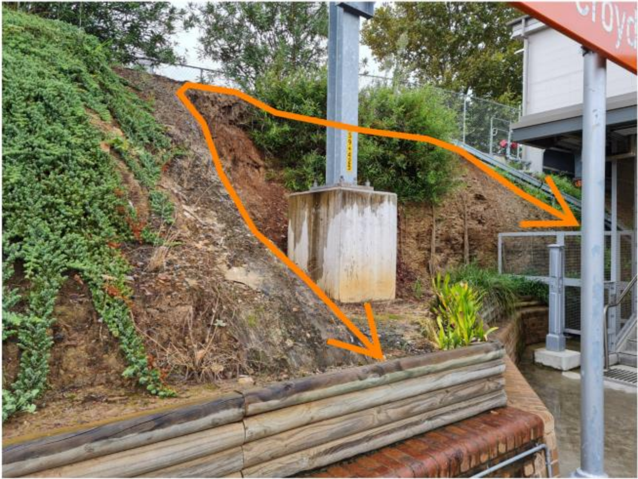
Figure 2-2 Photo of Eroded Cutting
