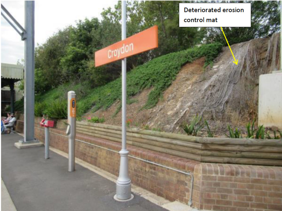
Photo 2: Failed section of the cutting
