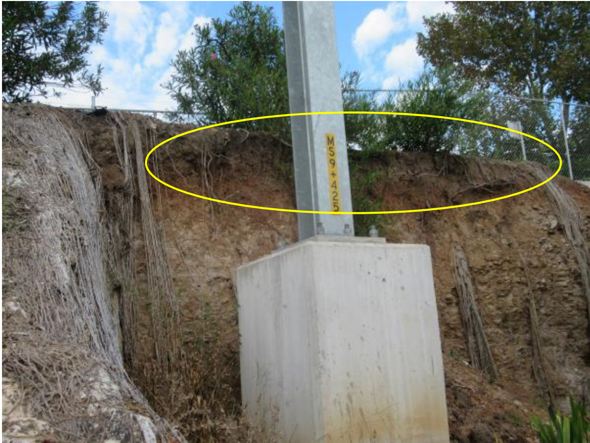
Photo 3: Undermined section of cutting at top
