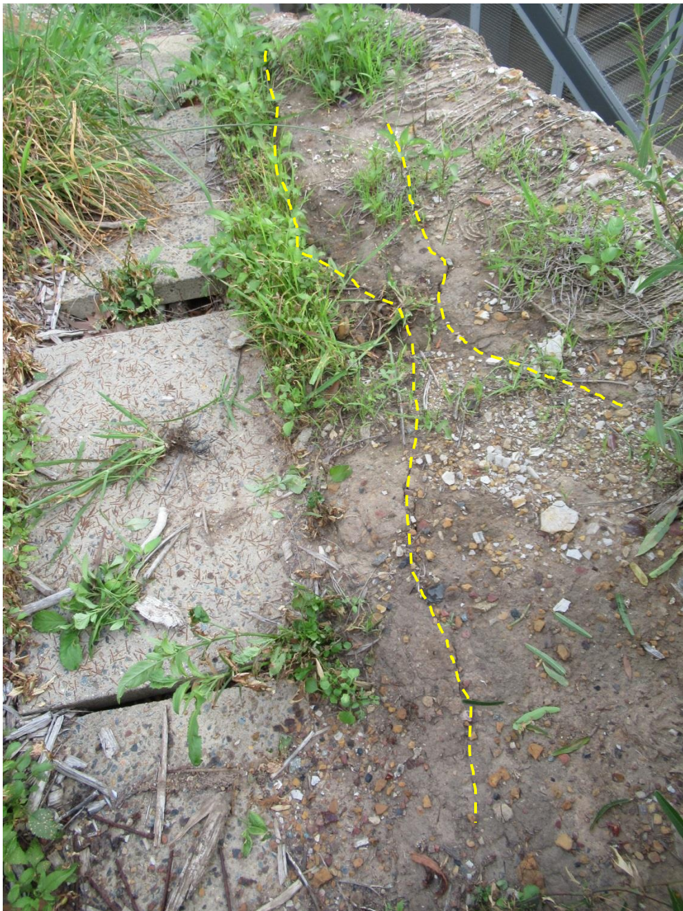
Photo 5: Typical tension cracks at top
