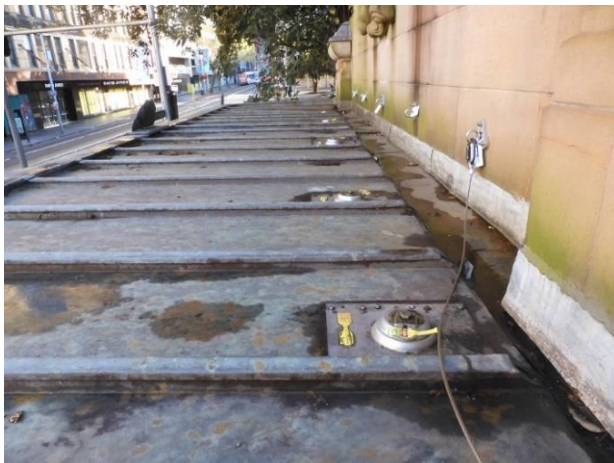
Figure 17: Batten roll copper roof cladding and copper box gutter to awning installed in the 1990s. Note roof access anchor locations, the fixings of which have penetrated the roof cladding.
