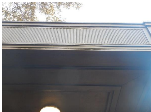
Figure 24: Minor damage to awning fascia
