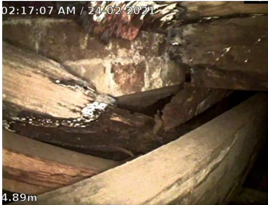
Figure 25: Still from CCTV video showing deteriorated awning roof framing
