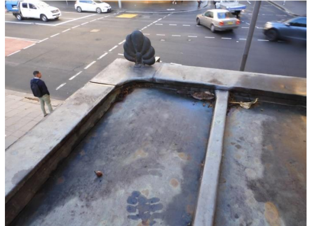
Figure 20: Corner of awning roof showing top of fascia cladding and copper acroteria
