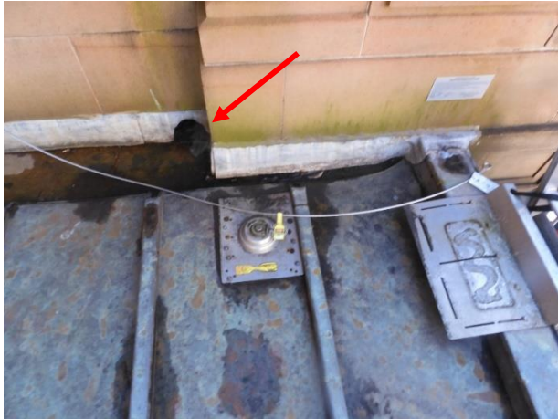
Figure 19: Horizontal box gutter outlet at southern end of roof created as part of 1990s roof and box gutter replacement. Ladder access bracket at right hand side
