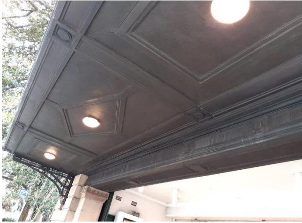
Figure 11: Original copper ceiling lining to awning. Note water staining to copper clad beam to the rear.
