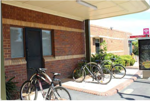
Figure 33: View of entry to office (left) with 1994 modifications matched to original brickwork.
