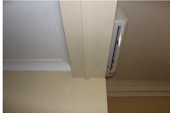
Figure 40: Air-conditioning unit and intersection between the original space and 1994 addition.
