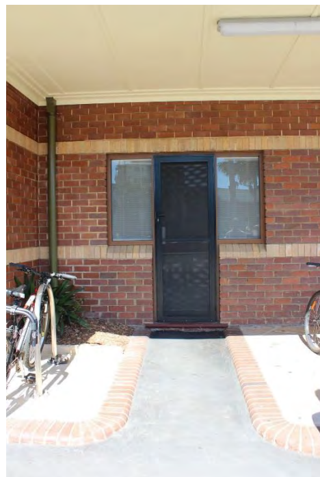
Figure 32: Entry to office showing modern aluminium windows and door, as well as 1994 paving elements.
