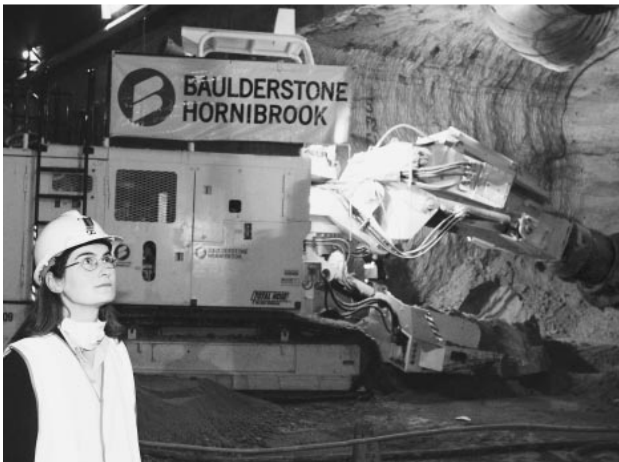
Construction of the Cross City Tunnel began in January 2003. The tunnel will be opened to traffic in 2005.
