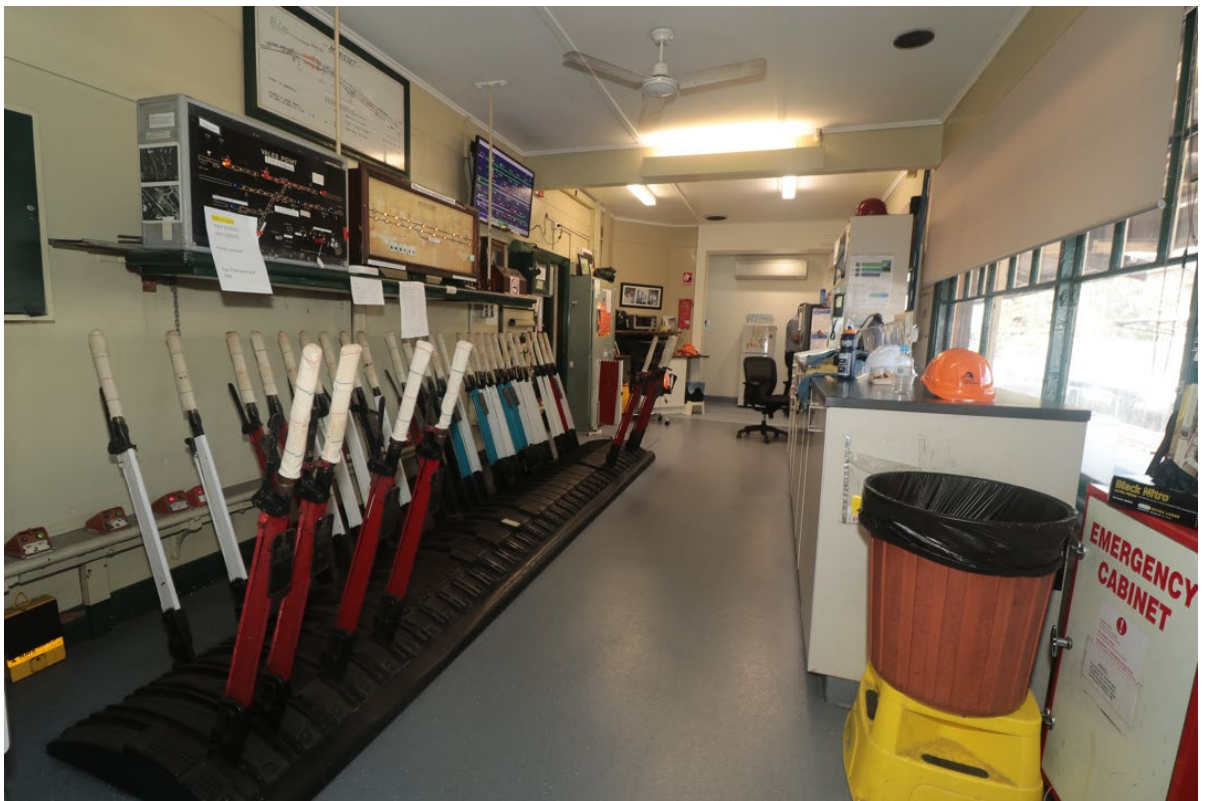
Figure 4-1: signal box interior. See also Figure 3-7
