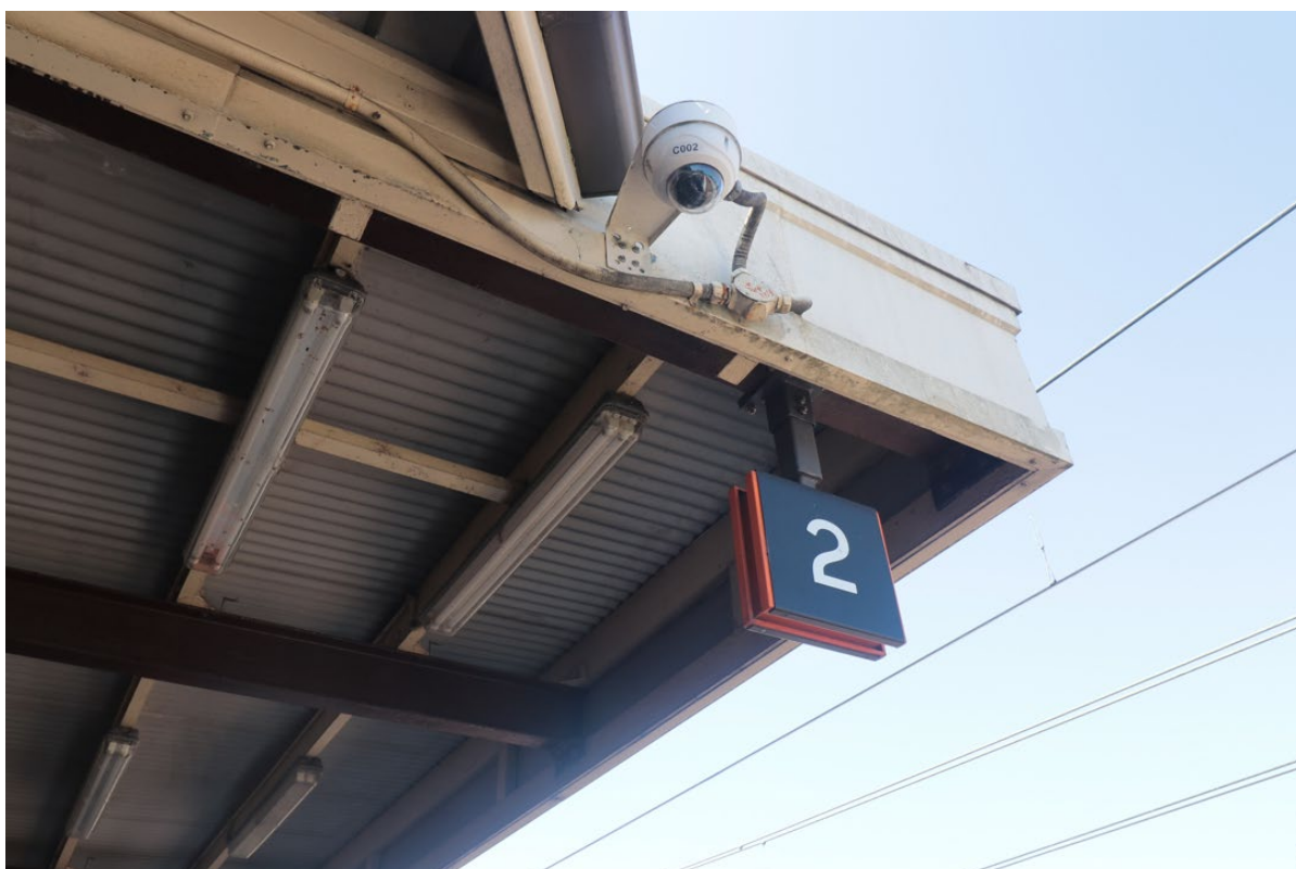
Figure 7-2: platform wayfinding signage with contemporary, sympathetic, bracket fixed with clamps
