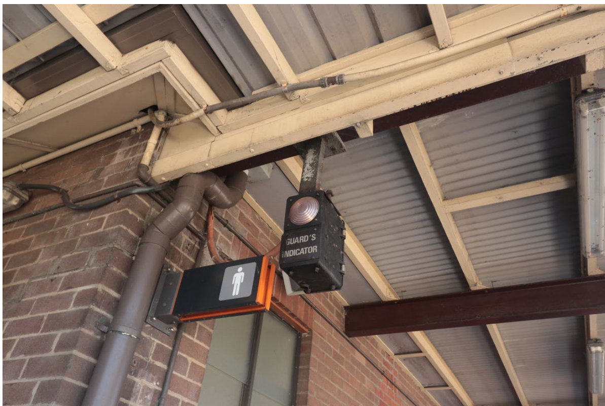
Figure 7-1: existing guard indicator with fresnel lens, to be replaced
