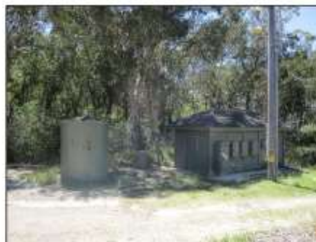
Figure 13. View east showing electrical substation and infrastructure within the rail corridor between Morisset Station and Vales Point.
