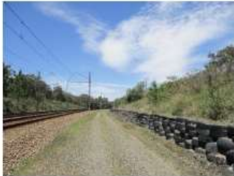
Figure 11. View north of retaining wall established to maintain cut of rail line.
