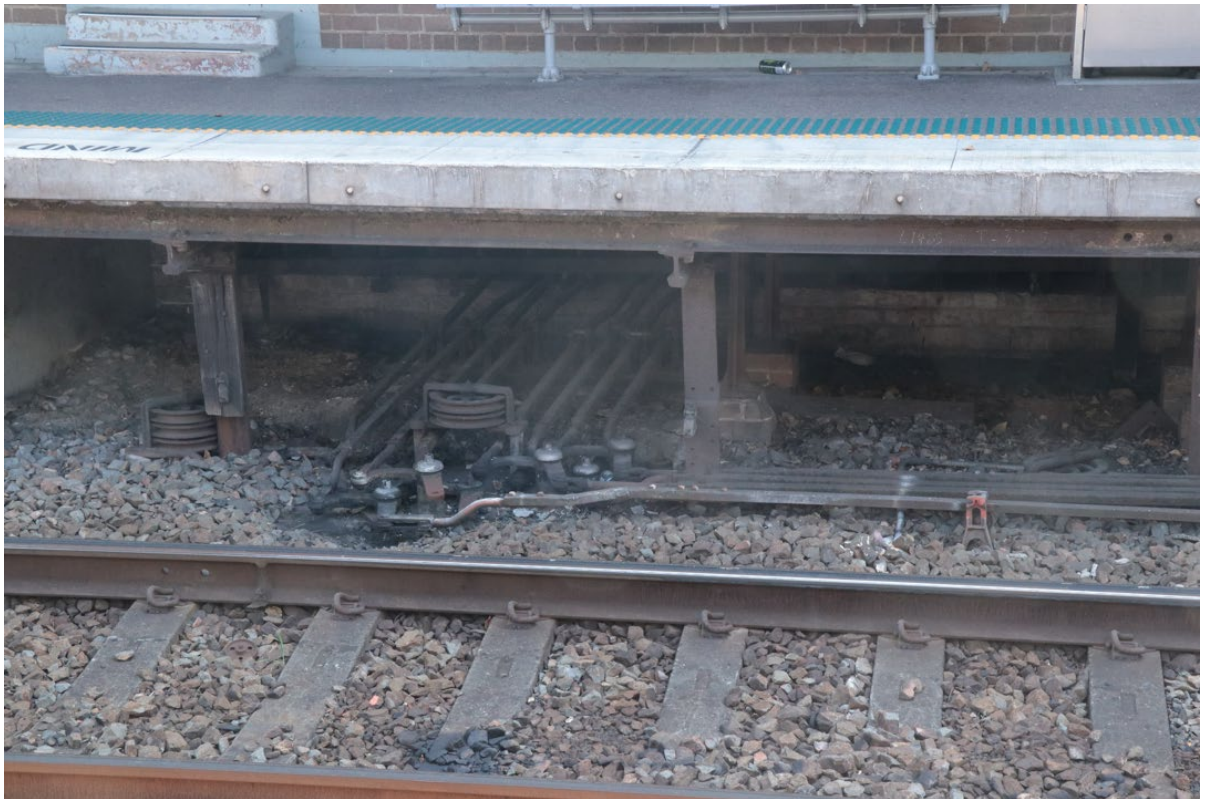
Figure 7-10: signal rods and pivots where they emerge from the underfloor of the Signal Room on Platform 2.
