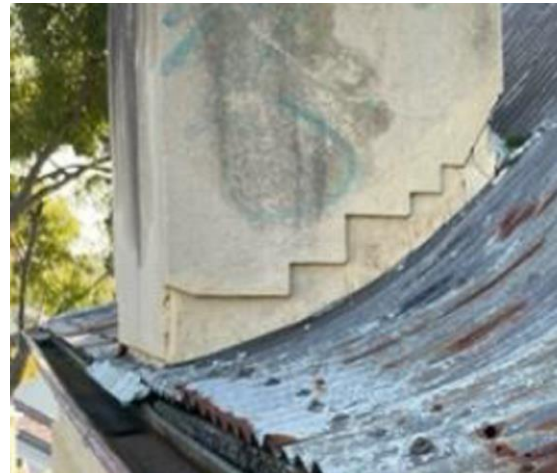
Figure 18: Evidence of poor flashings (OCP, 2023)
