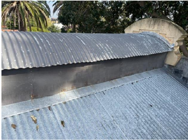
Figure 19: Curved dome lantern: evidence of lost detailing – likely originally timber louvred and glazed (OCP, 2023)
