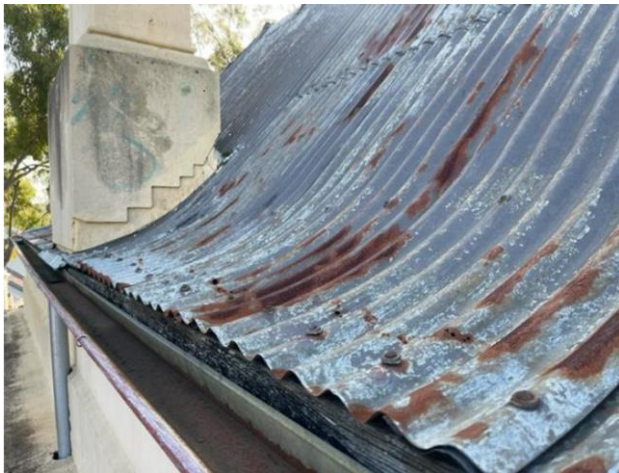
Figure 17: Existing corroded roof sheeting (OCP, 2023)
