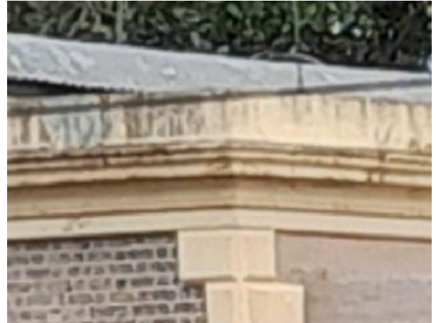
Figure 20: Parapets in poor condition (OCP, 2023)
