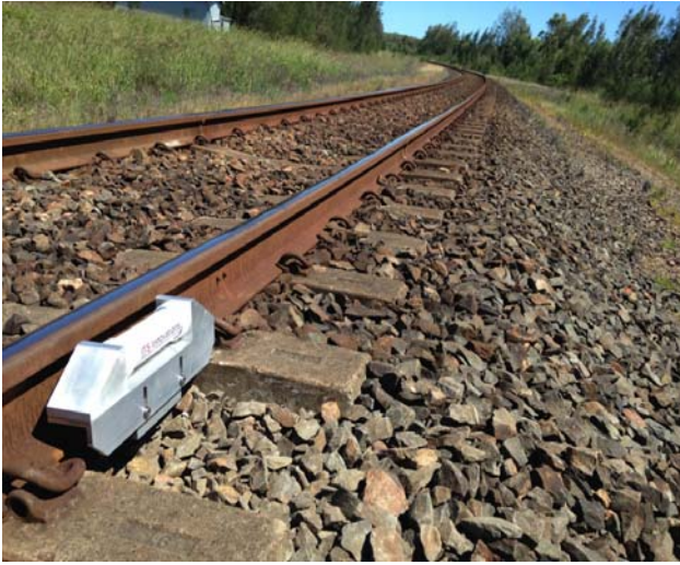
ITS Innovations level crossing warning system installation in NSW
