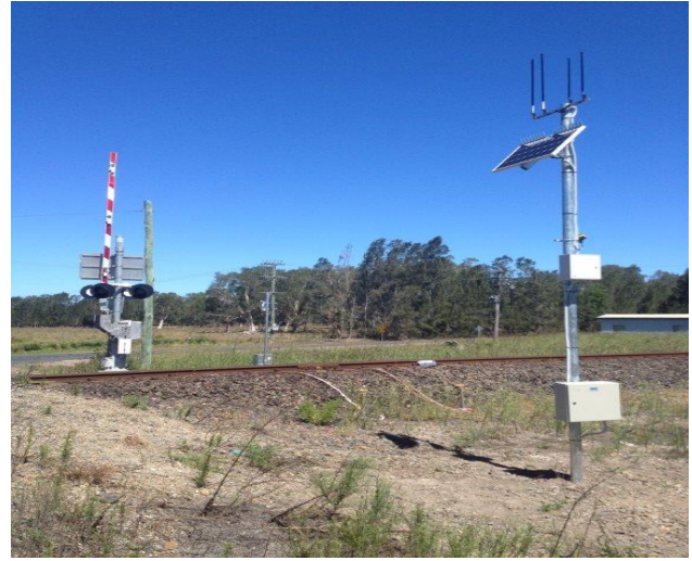
ITS Innovations Control Location
