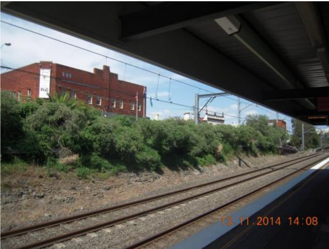
Plate 8 Dense environmental weed growth within rail corridor along Hennessy Street
