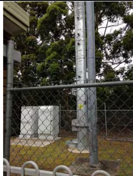
Photograph 10: Base Transceiver Station
