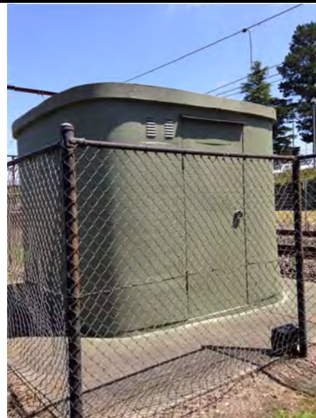
Photograph 10: Relay and Signalling Hut (637B)
