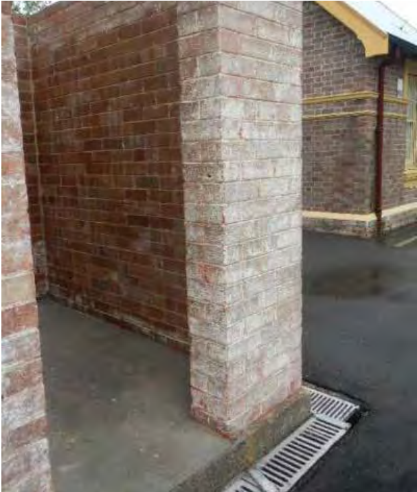
Image 9 Slab, screen wall and curtain walls to the south of the Men's Toilet proposed to be removed
