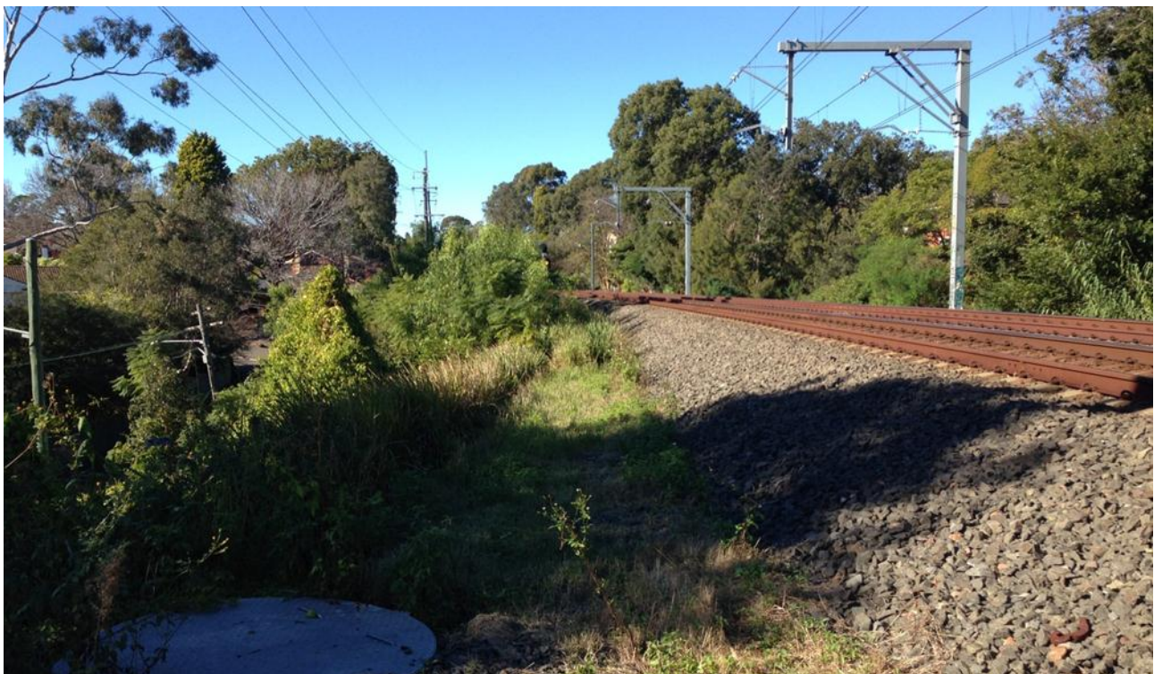
Figure 1.9 Typical example of the southern end of the proposal site for the installation of the new combined services route, to the north of Clanville Road
