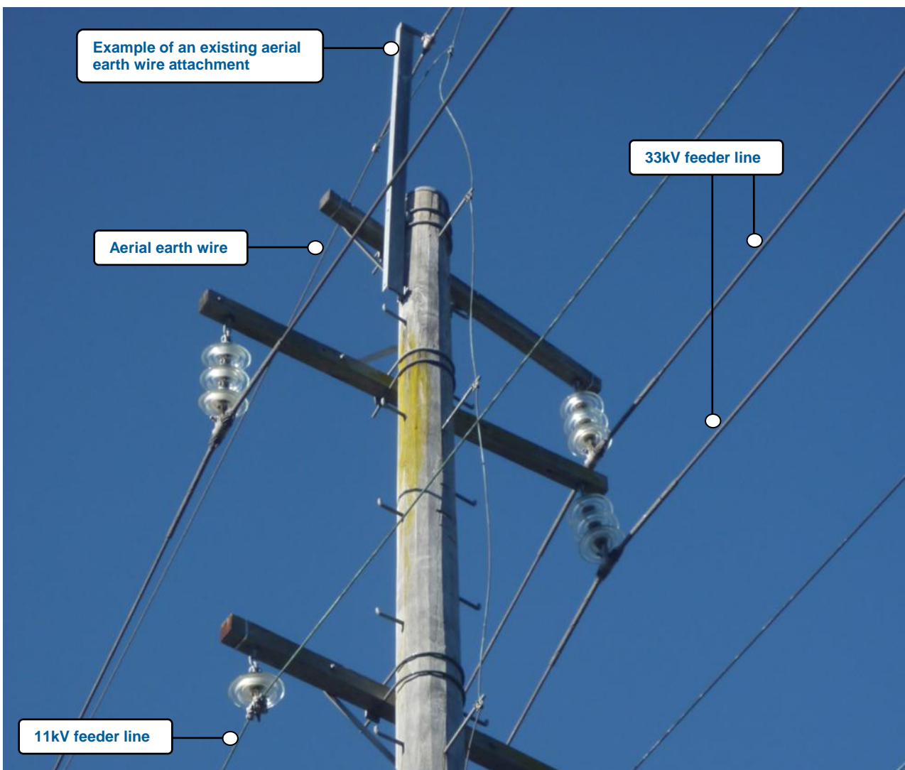
Figure 5.7 Example of a typical aerial earth wire arrangement on the top of an existing power pole
