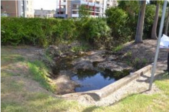
Figure 23: Drain in the north-eastern part of the proposed car park at Site 2 facing north-west
