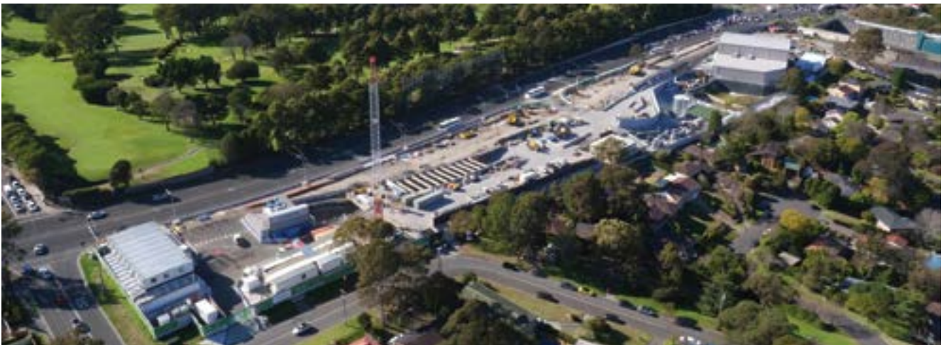
NorthConnex southern interchange compound at Pennant Hills Road and the Hills M2 Motorway
