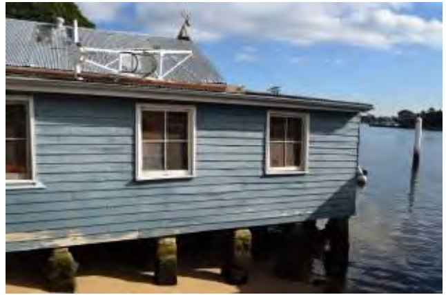
Figure 11: A general view of the eastern façade of the Abbotsford Point Boatshed, adjacent to the wharf.
