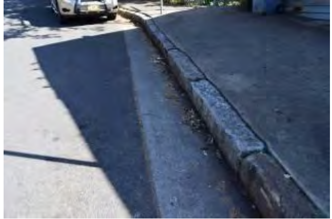
Figure 14: A closeup view of the sandstone kerbing along Great North Road, facing west.
