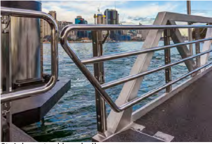
Stainless steel handrails
