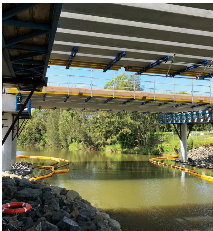
All 230 planks have been installed on the bridge over Macquarie Rivulet - May 2020
