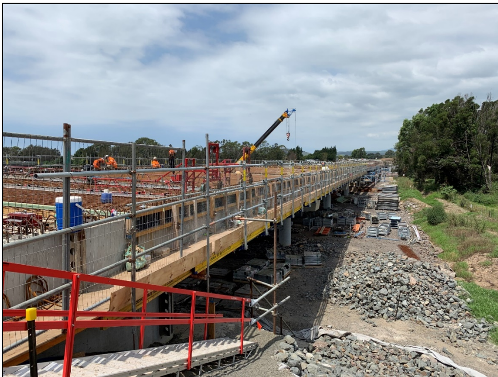
Photo 1: View of the construction activities associated with the new bridge (Bridge No. 5) over Macquarie Rivulet at Yallah during January 2020. Works at this location have been conducted in accordance with the approval issued by the Civil Aviation Safety Authority (CASA) Air Navigation, Airspace and Aerodromes Branch on 05 December 2019.
