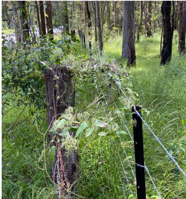
Figure 33 Overgrown section of new fencing adjacent to disused timber fencing. Communications trenching adjacent to fence alignment.
