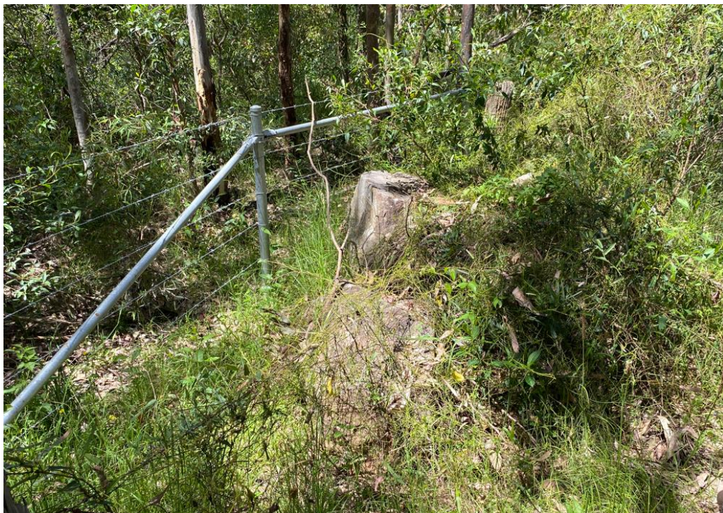
Figure 44 Overgrown stockpile of concrete and pavement materials adjacent to newly installed fence.
