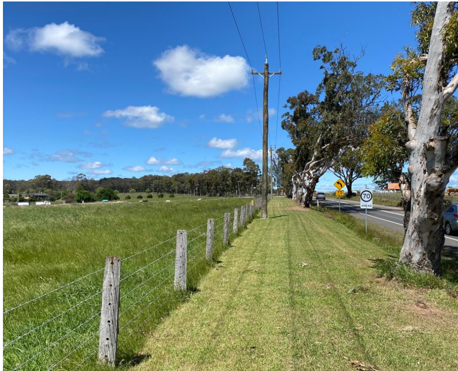
Figure 10 Electrical overhead route along fence line. Mown access for maintenance.
