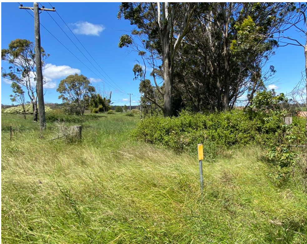
Figure 7 Communication trench markers along fence alignment. Electrical maintenance track adjacent to fencing
