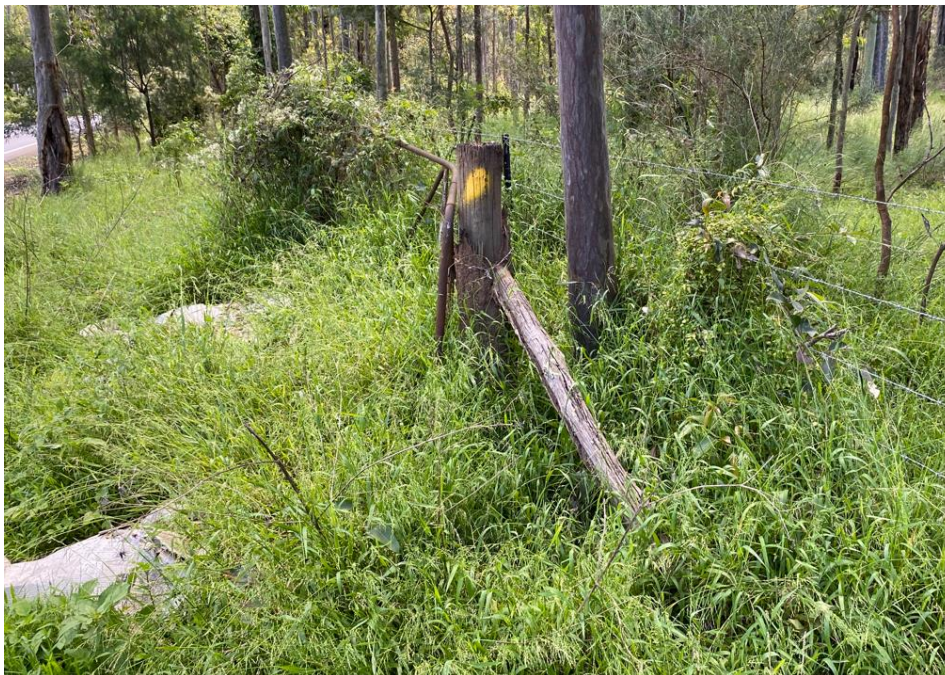
Figure 32 New fencing installed adjacent to previous fence. Disused gate and fence posts left in place. Dumped rubbish along fence line.
