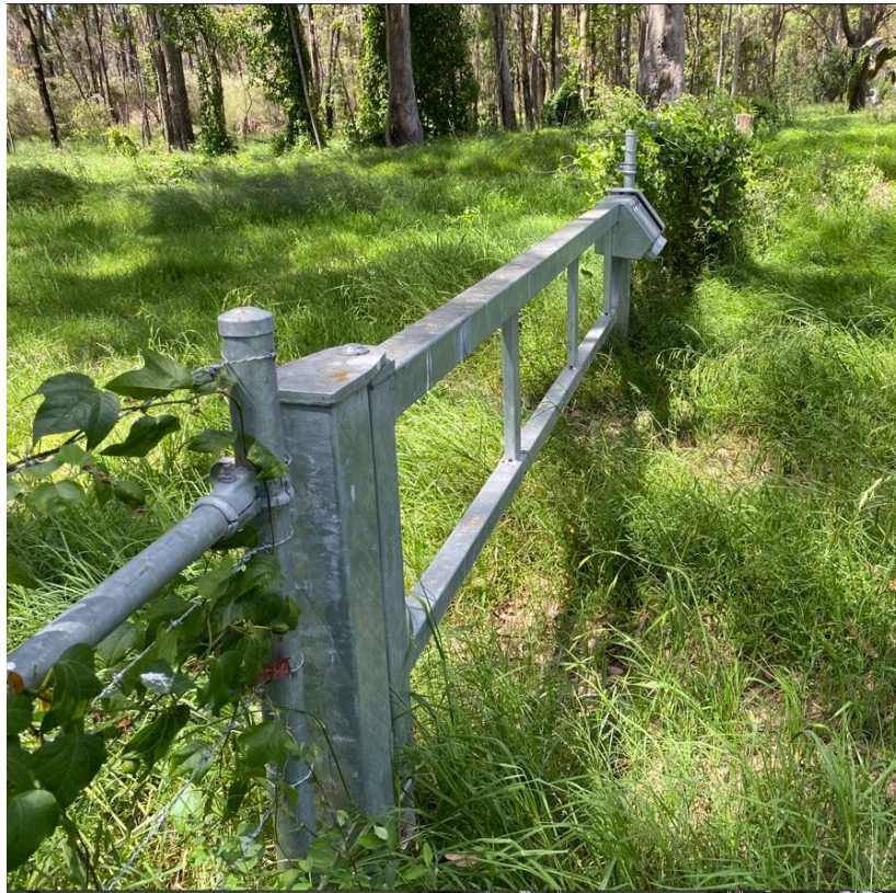
Figure 25 Electrical maintenance and bushfire access gate overgrown. Communications trenching along fence route.
