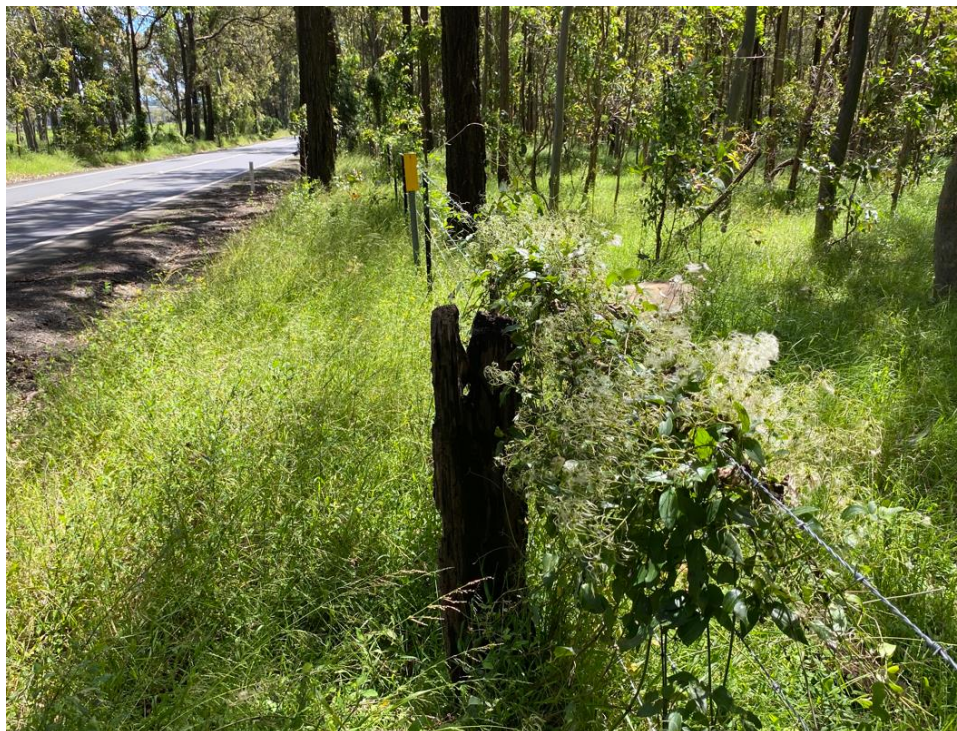
Figure 34 Communications marker post indicates adjacent service trenching. New fencing installed adjacent to disused timber fencing.
