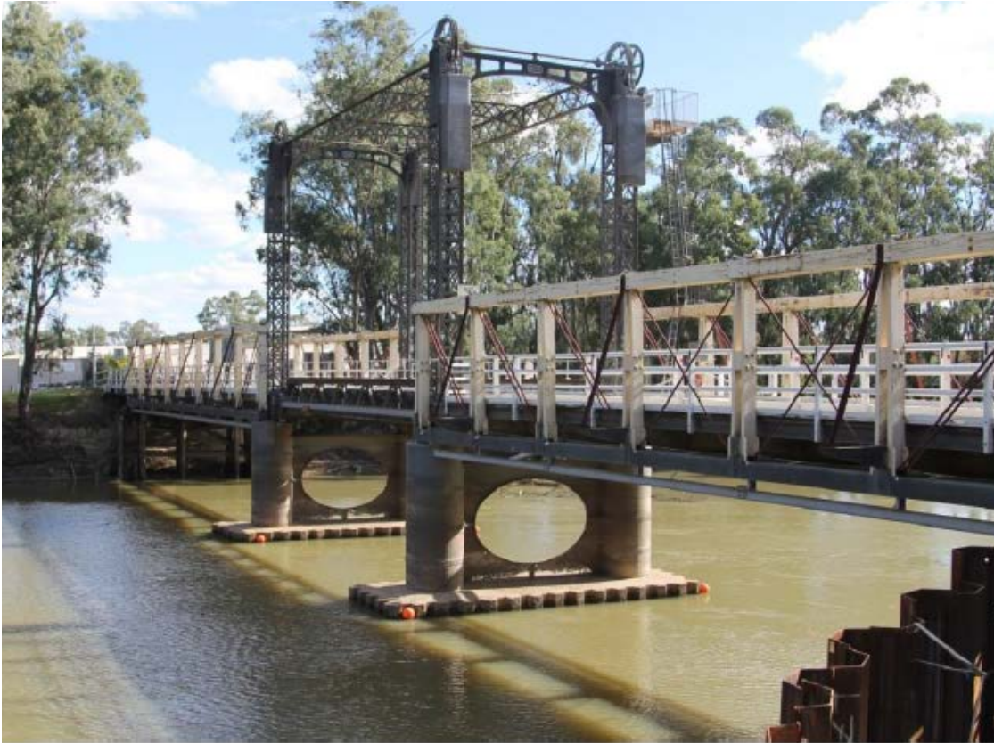
Figure 2 - Barham Bridge looking south west, showing deterioration of the pier webbing on both river piers (Source: Roads and Maritime)
