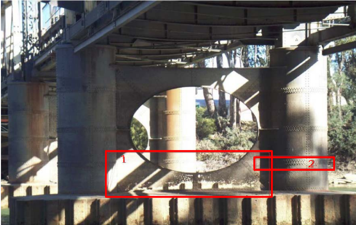
Figure 4 – Barham Bridge: 1. Pier webbing corrosion. 2 Caisson splice repair location (Source: Roads and Maritime)
