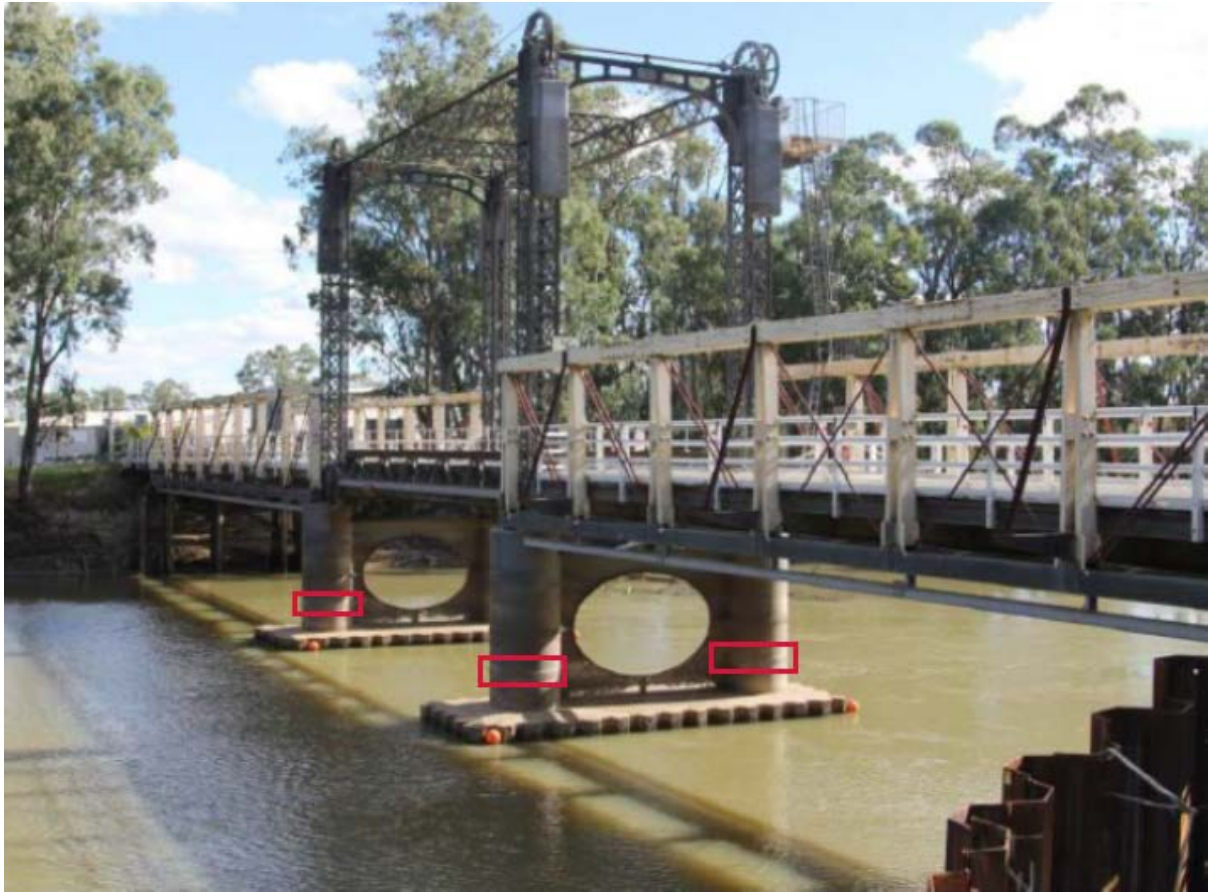
Figure 3-2: Barham Bridge looking south west showing the location of the caisson repairs
