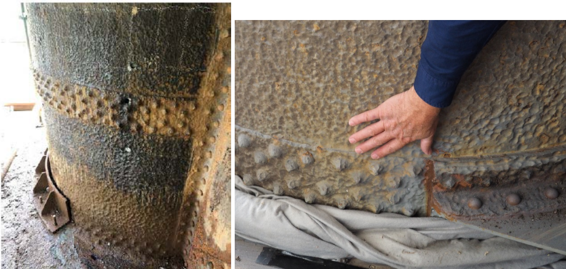
Figure 3 - Showing corrosion at caisson splice (Source: Roads and Maritime)
