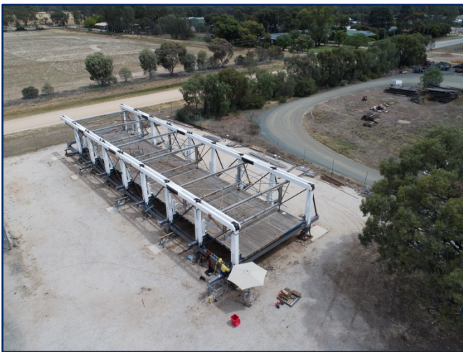
The new bridge trusses were built in site compounds in Barham and Koondrook.
