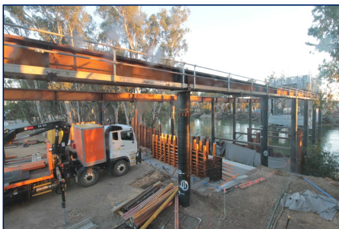
The lift and skate gantry on the Victorian side of the bridge.
