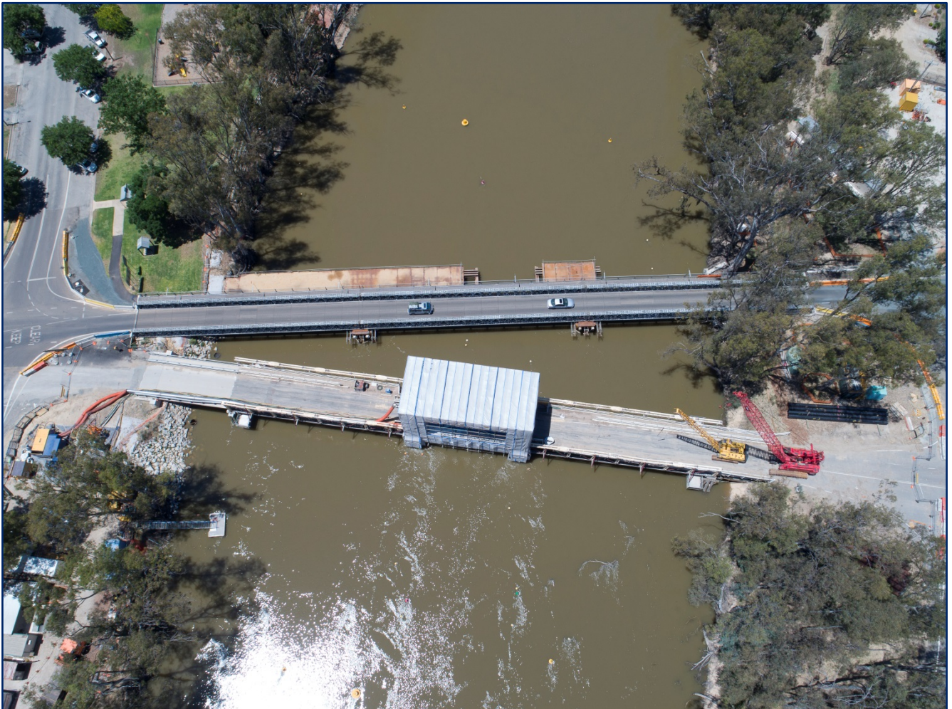
An aerial view of the work site from November 2017. This photo shows the containment around the lift span to avoid polluting the river.
