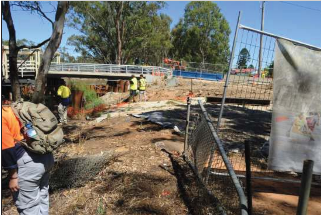
Plate 5: Disturbance east of the Barham Bridge, facing 280° (Photo: B. Grinter 12/12/2014)
