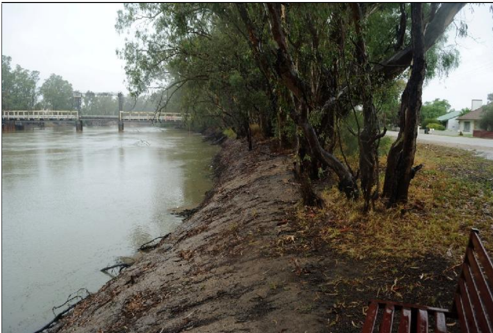
Plate 2: Eroded river bank, facing 130° (Photo: J.Bell 13/1/15)
