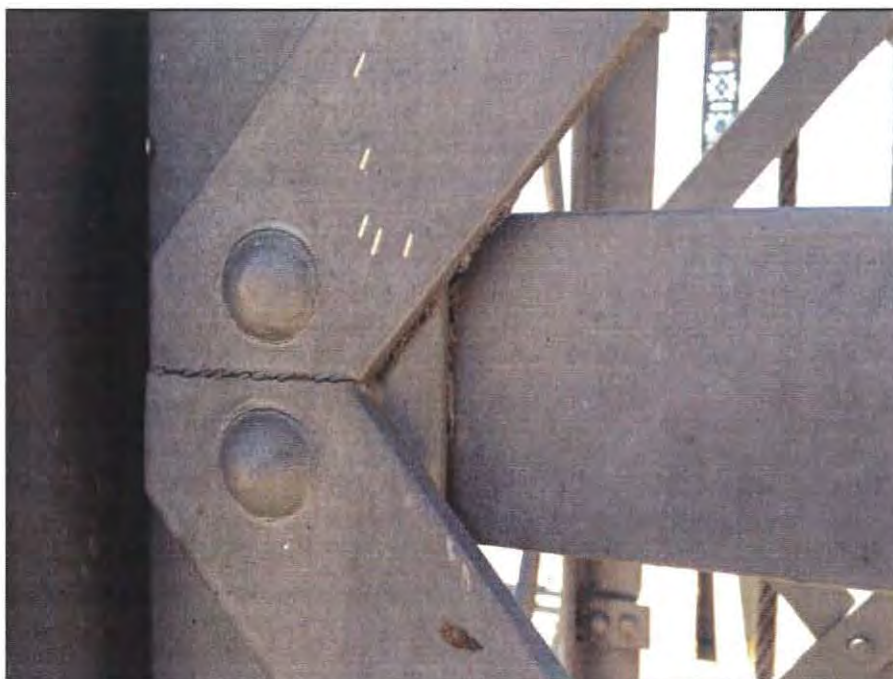
Plate 4: Detailed view of silver-grey paint on metal lift-span bridge elements where sample PS-7 was collected. Paint was noted to be in fair to poor condition and laboratory analysis indicated that lead was present.
