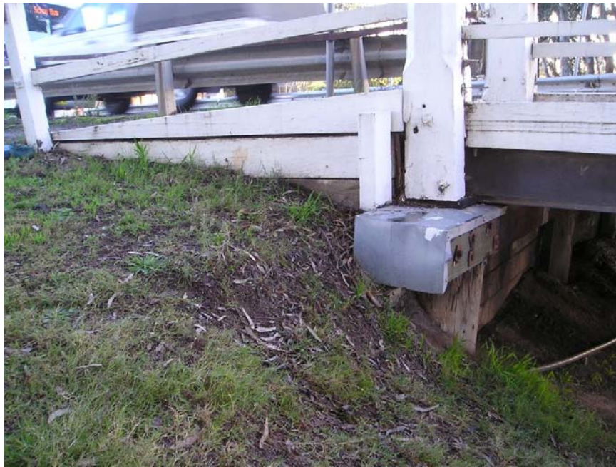
Figure 16: View of Abutment B detailing its low clearance above the river bank.
