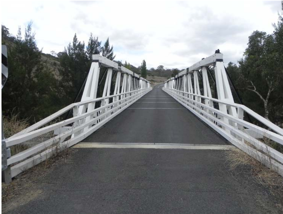
Figure 31: View of Wallaby Rocks Bridge, north of Bathurst following completion of upgrading works in 2010 showing SLT decking and steel guardrails.
