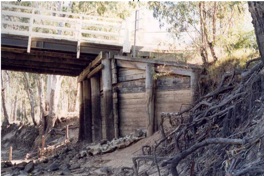
Figure 15: View of Abutment A looking west in 2004 prior to replacement in 2013. Stones from the original spill through abutment can be seen at the base.
