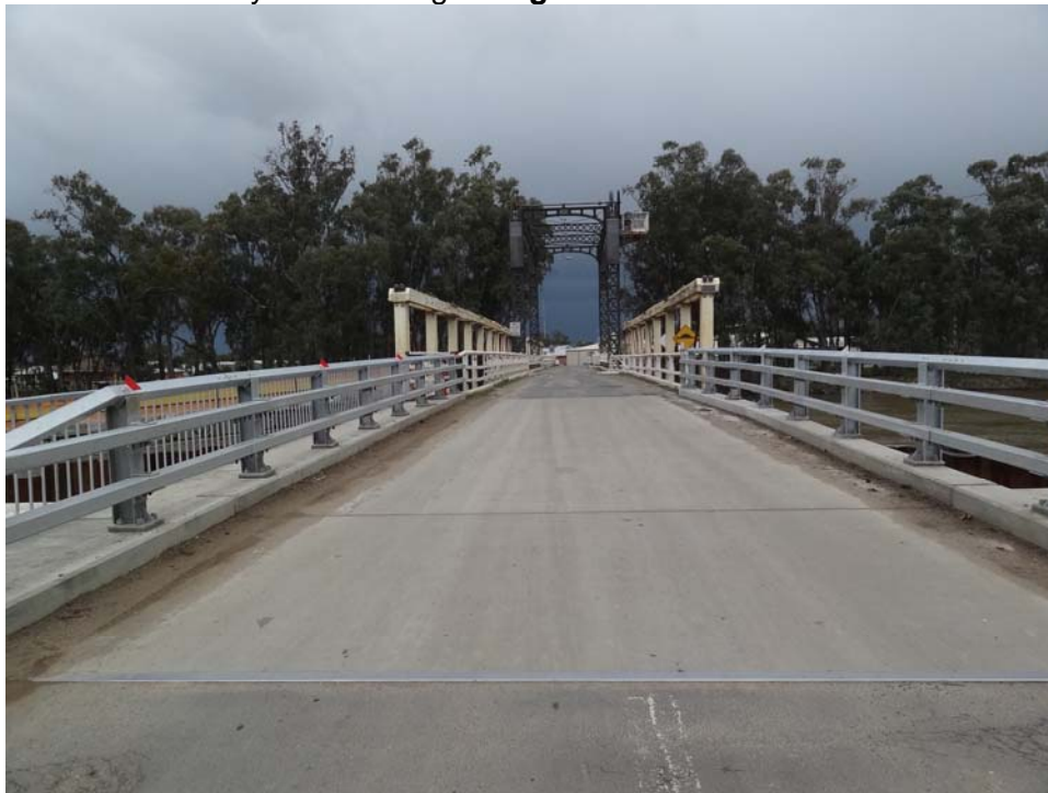
Figure 30: View completed NSW approach span (span 1) of Barham Bridge in March 2014 prior to painting of barrier railing white.
