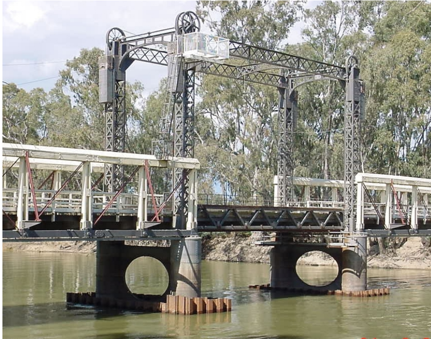
Figure 19: View of the Warren truss of the lift span on the upstream side.
