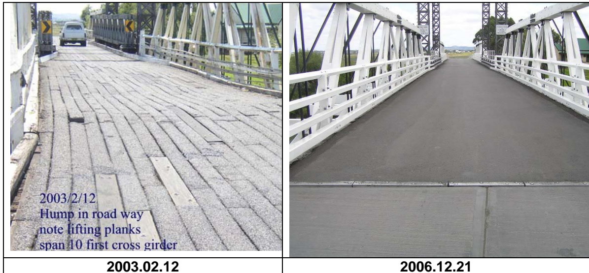
Figure 27: Two views of capacity upgrade of Hinton Bridge, detailing the change from timber planks to an SLT decking system topped with a rubberised bitumen seal.
