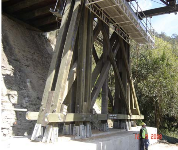
Figure 29: View of Pier 4 of St Albans Bridge detailing pilecap and steel shoes at base of timber trestle. A tall spill through abutment is visible at left.
