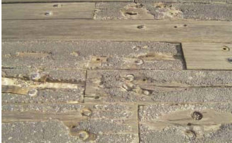
Figure 25: Detailed view of deck detailing its poor condition with splits and decayed timber.
