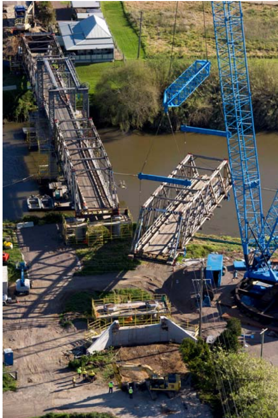
Figure 33: Truss being removed from Dunmore Bridge in 2013 prior to a replacement truss being manoeuvred into position.
