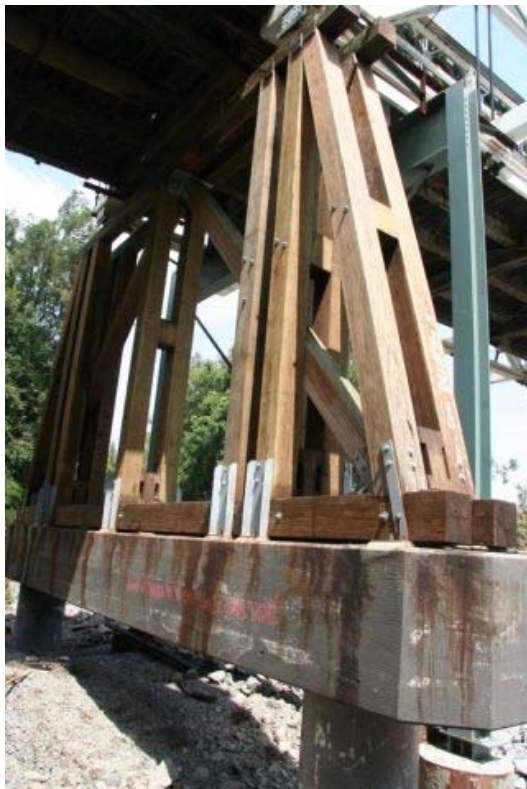
Figure 30: View of Pier 3 of Coorei Bridge detailing pilecap and steel shoes at base of timber trestle. The capwale is just visible at the top of the pier.
