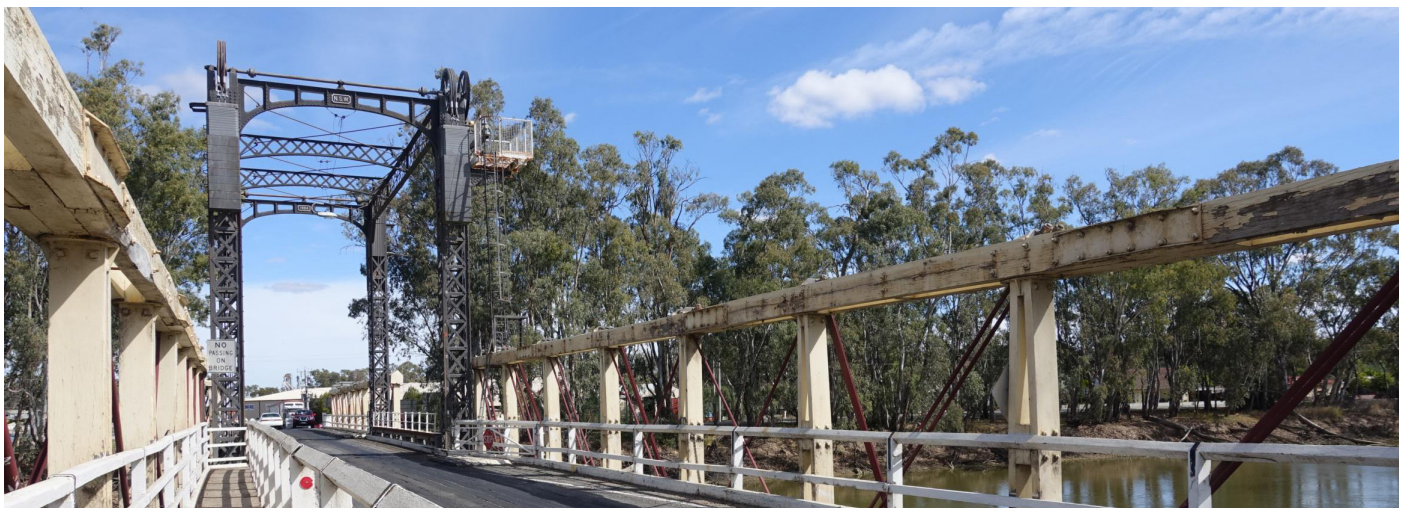
Figure 6: View looking towards the tower of the lifting span that forms an important element of the bridge
