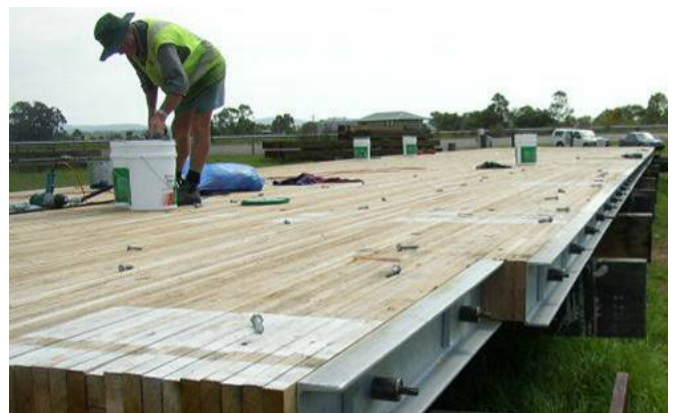
Figure 33: Bridge timber deck construction. The picnic table would use a similar construction approach to illustrate this methodology
