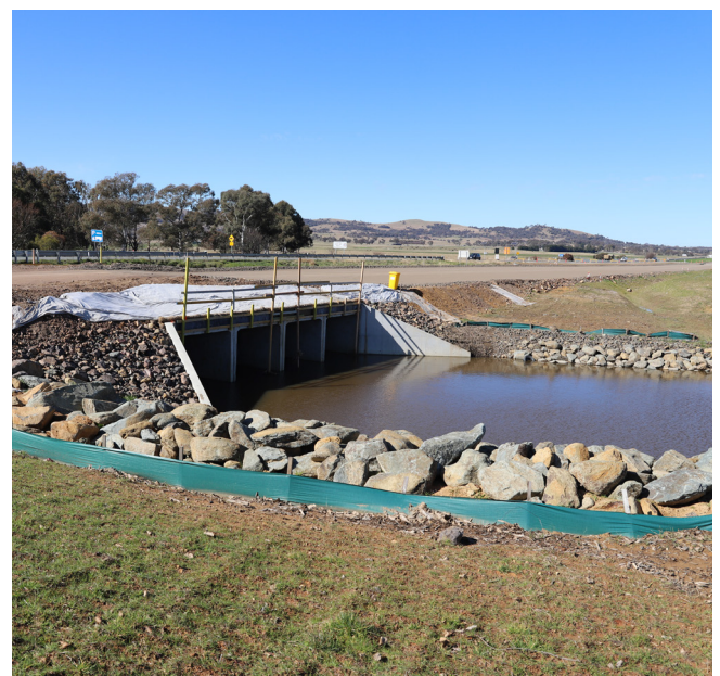
Drainage work has been completed under the new northern carriageway at Gooromon Ponds.
