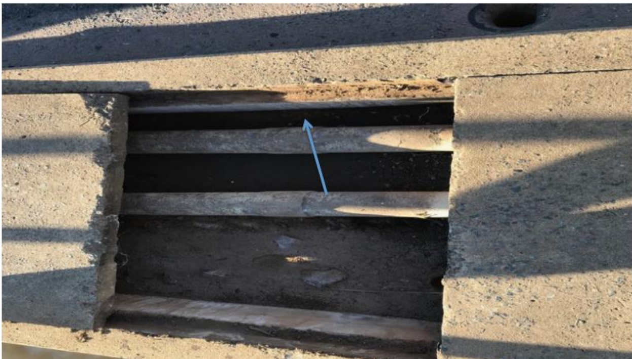
Figure 6-16: Friable asbestos detected within loose fibre bundle within the underside of the concrete slab.
