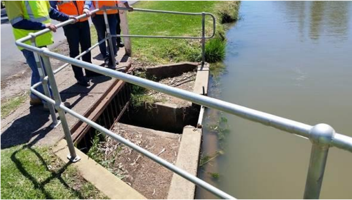
Figure 6-15: Water level control structure downstream of Camp Street Bridge, Lake Forbes at Sherriff Street.
