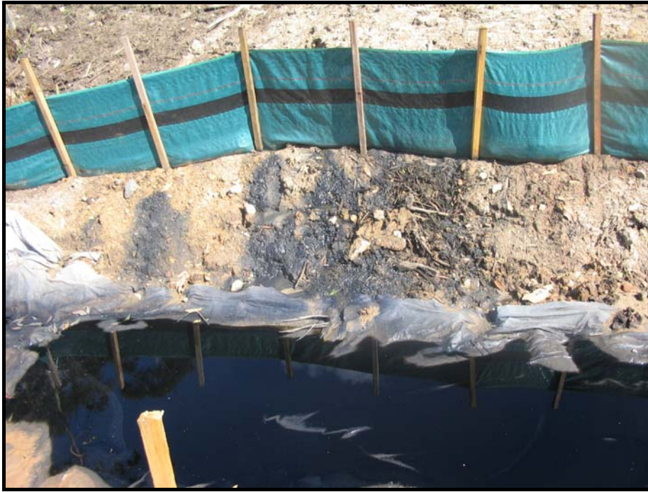
Plate 5: Tannins in a drainage line generated from very thickly applied mulch on the batter above. Note that the sedimentation fence is not effective in treating the tannins.
