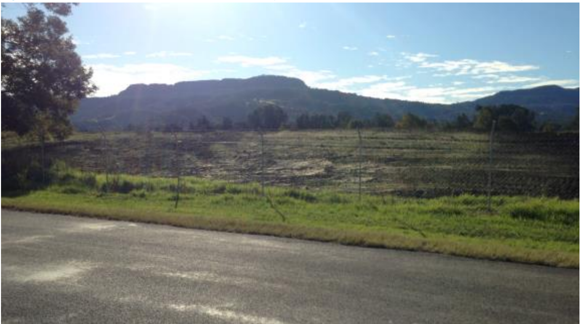
Figure 3-6: Earthworks continue behind the recently stabilised noise mound on North Street, Berry.
