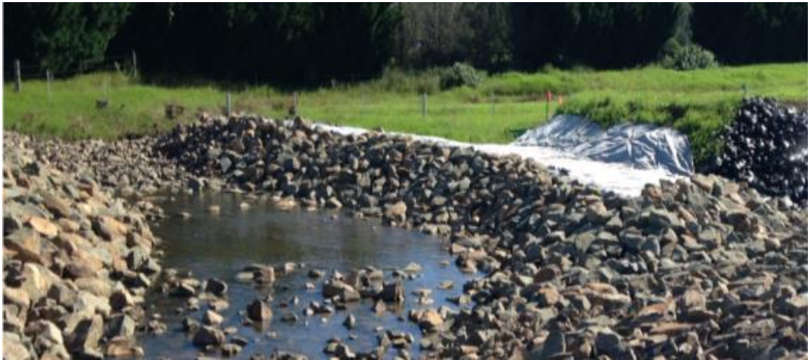
Figure 3-3: Clean water diversion installed at project chainage 9800 to allow the designed drainage culverts to be completed but still maintaining upstream downstream clean water connectivity.
