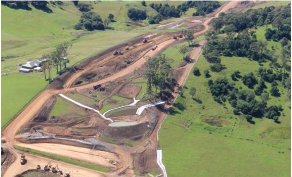
Figure 3-5: Sediment basin at Cut 2b, constructed for capturing sediment laden site runoff.
