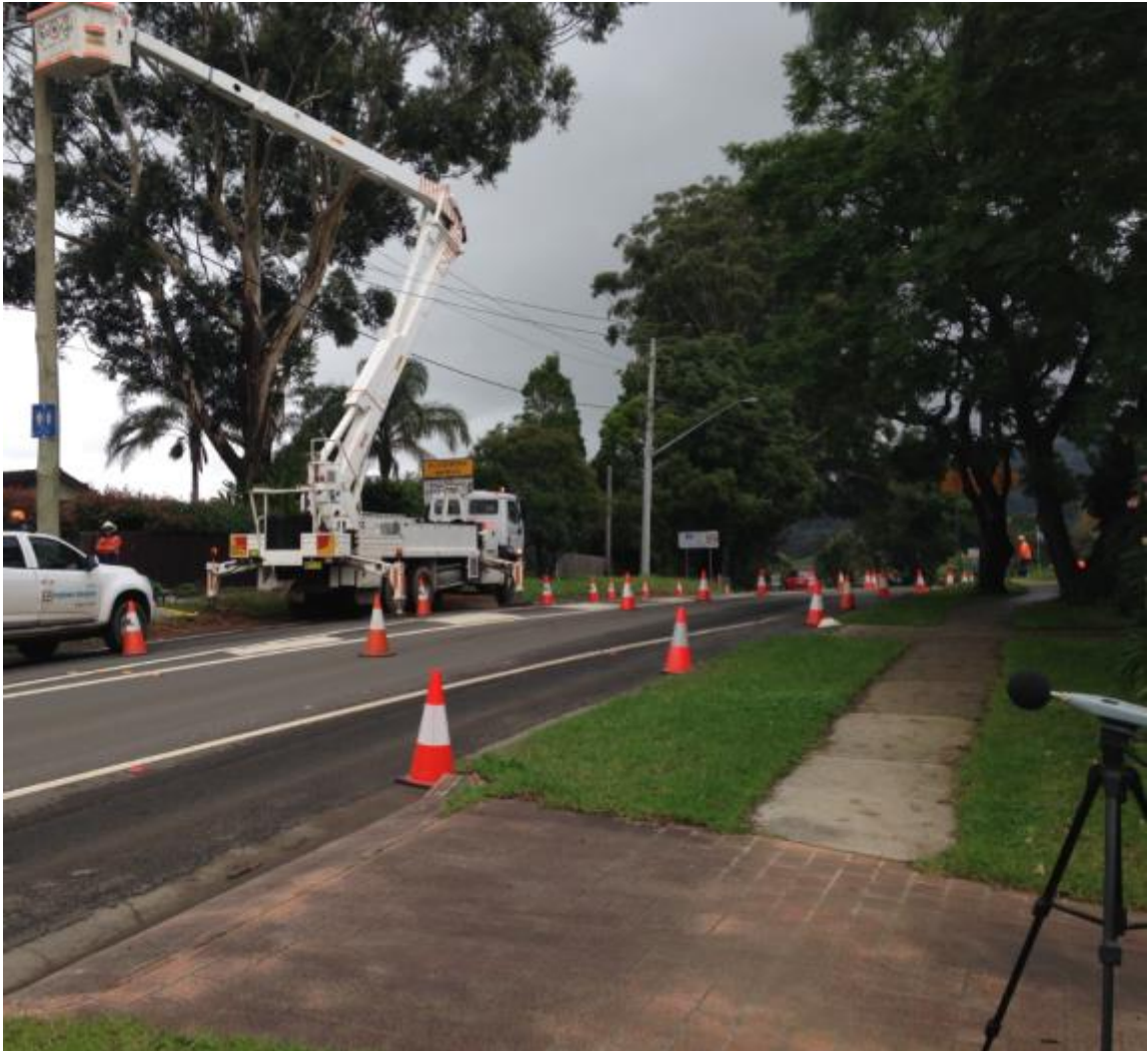
Figure 4-5: Out of hours inspection during services installation works at Kangaroo Valley Road Berry
