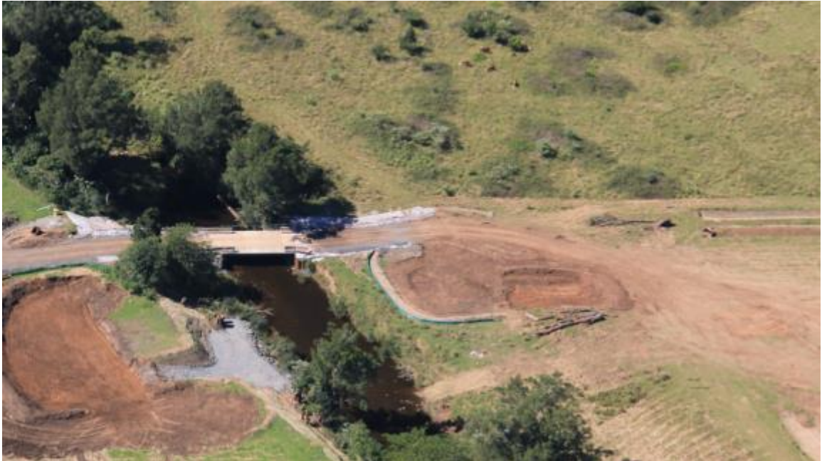
Figure 3-7: Temporary Bridge at Broughton Creek crossing no.2, adjacent to the new highway bridge site.
