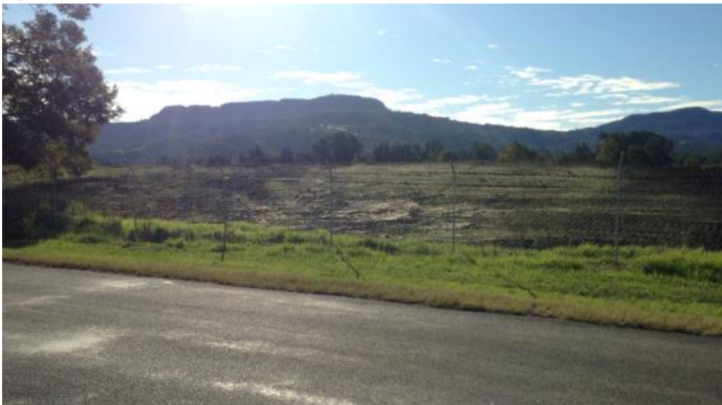
Figure 2-4: Earthworks continue behind the recently stabilised noise mound on North Street, Berry.
