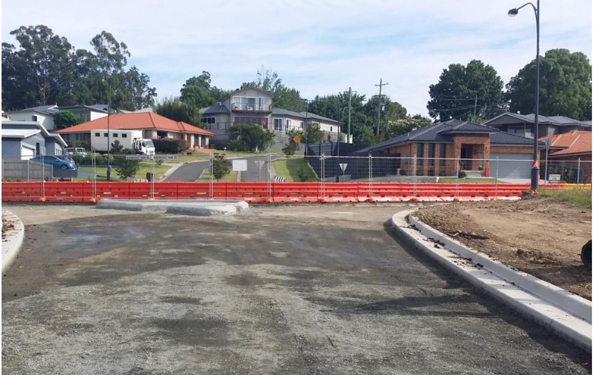
Figure 2-2: Temporary fencing during the construction of the new Hitchcocks lane connects to Huntingdale Park Drive, Berry.
