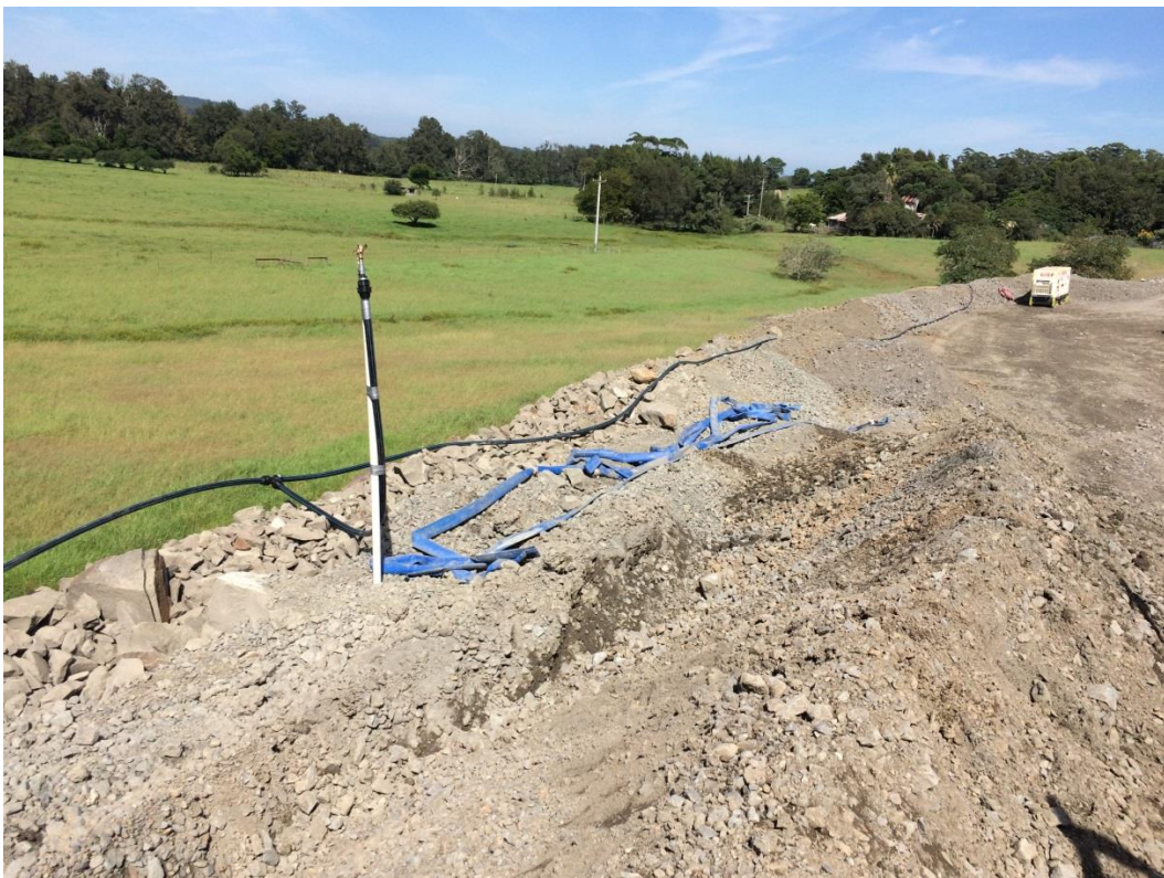
Figure 5-5: Additional sprinklers were installed at Austral park crushing compound. The aim was to keep material wet and reduce the potential for dust.
