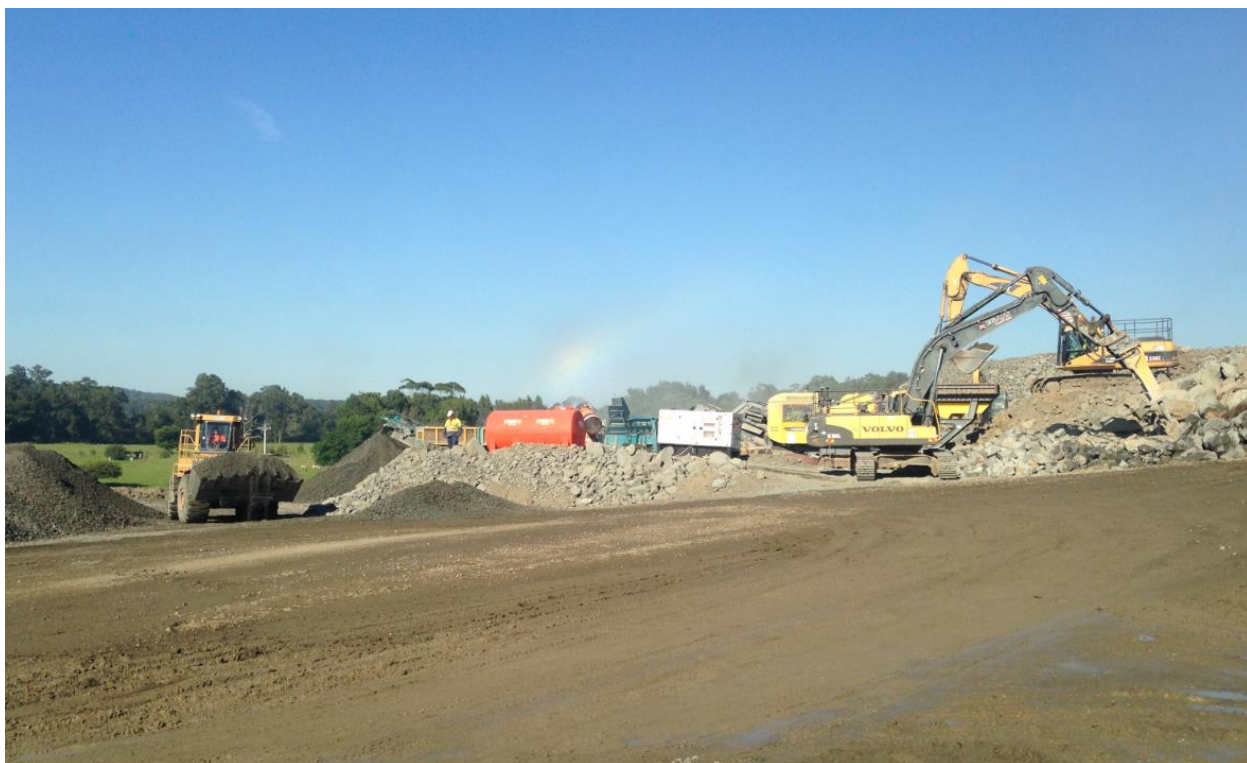
Figure 5-3: Water misting systems installed at the crushing compound site, Austral Park Rd, Broughton.
