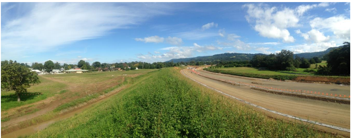
Figure 2-5: Earthworks continue behind the recently stabilised noise mound on North Street, Berry.
