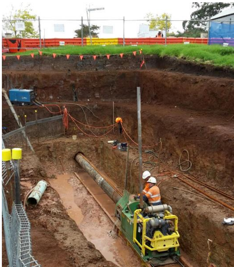
Figure 2-1: Under boring works for a new water main under Kangaroo Valley Road, Berry.
