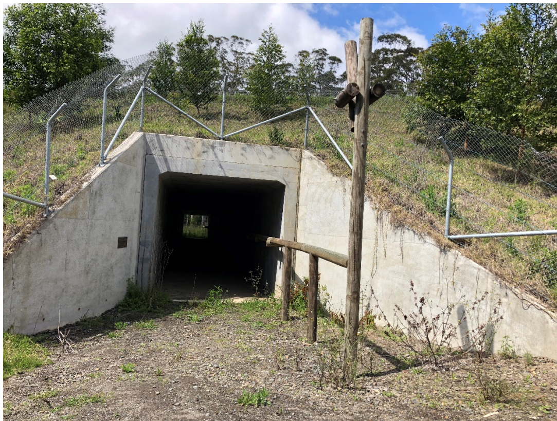
Figure 2-1: Fauna underpass complete with fauna furniture
