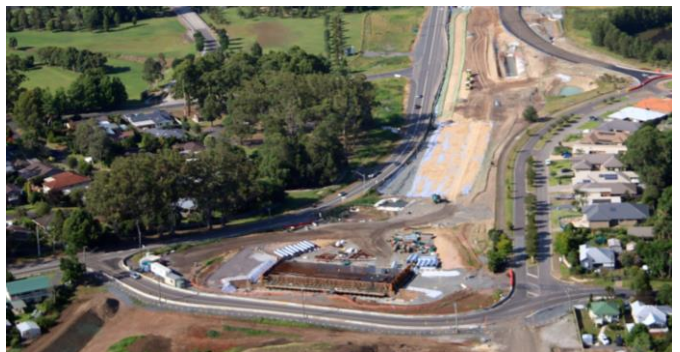
Aerial view of work to build the new Kangaroo Valley Road interchange, looking south west (December 2015)
