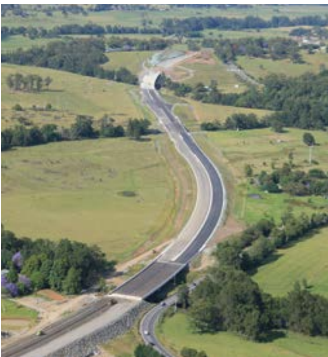
New highway lanes and bridge being built near Broughton Creek, looking south towards Berry
