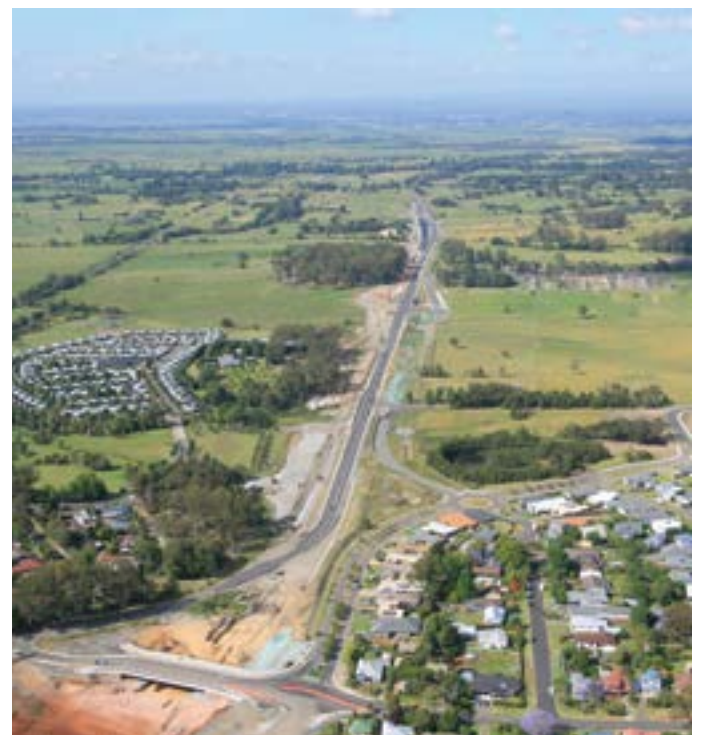
Kangaroo Valley Road bridge and new lanes being built, looking south towards Bomaderry
