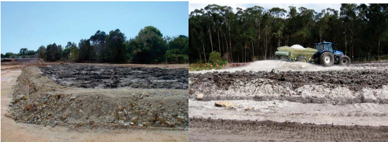
Photograph 1 Bunded treatment area for ASM and lime application
