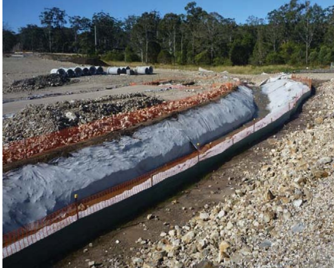
Figure 3. A geofabric lined temporary clean water diversion traversing a work zone during installation of cross drainage. The geofabric has been anchored at the top with star pickets at regular intervals. The star pickets are also integral to sediment fencing preventing sediment from entering the channel along the length of the diversion. Within the channel larger rock is used to aid in energy dissipation. Orange safety fencing effectively delineates the diversion and allows.
