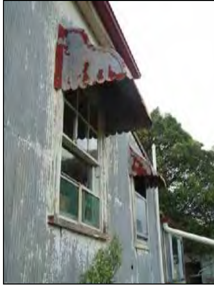
Figure G.165 Detail of awnings and corrugated iron cladding on N side of building
