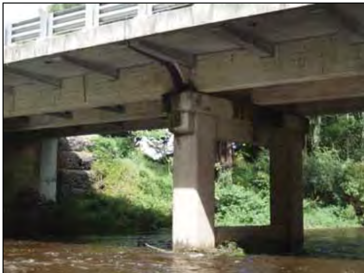
Figure G.138 General view of central pier, longitudinal beams and cantilever supports for widened deck
