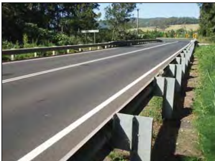
Figure G.139 General view of road top and approaches to bridge, looking NE
