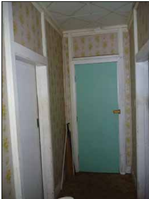
Figure G.104 View along central hall toward front door, showing exposed framing around doors
