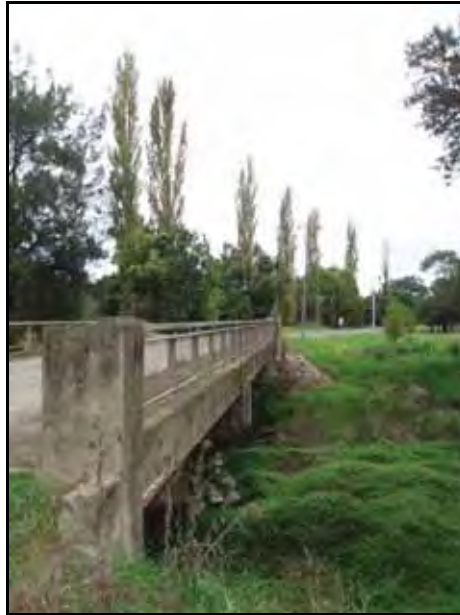
Figure G.222 General view of poplar avenue, looking S from the bridge over Bundewallah Creek
