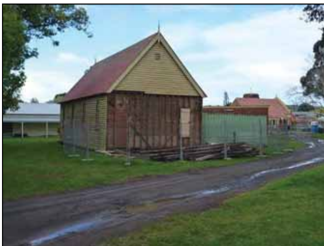
Figure G.186 Detail of demolition of skillion roofed addition to rear of chapel prior to relocation of main building (October 2011)
