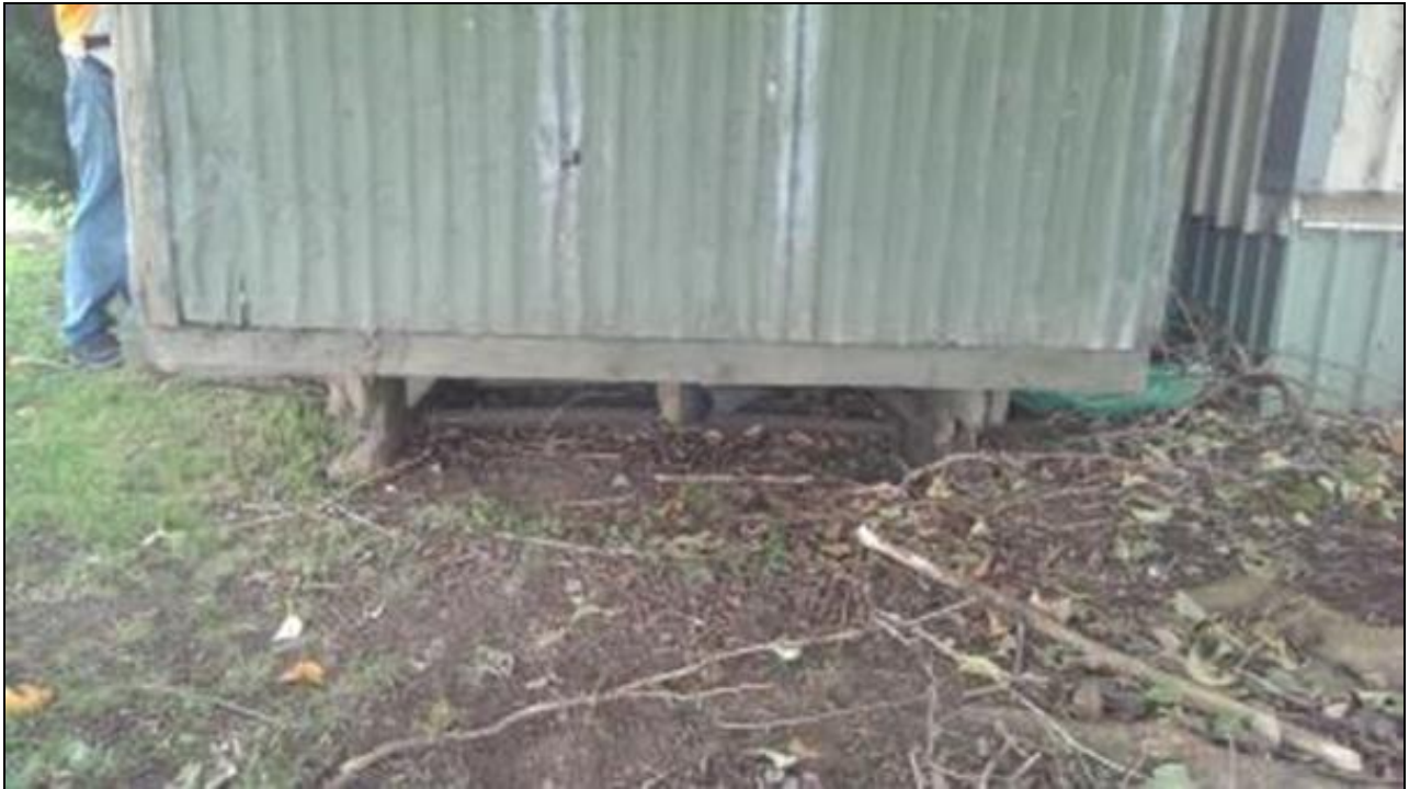
Plate 3: Detail of timber supports of skid mounted shed (G2B H60). Source: Biosis 2014
