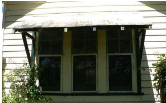
P1230584 Kitchen window hood
